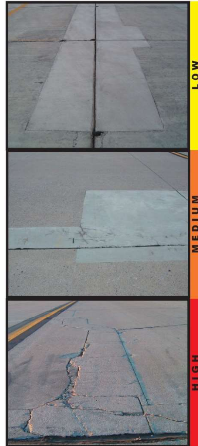
Figure C.15: PCC Large Patch.
