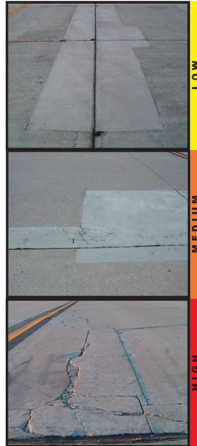
Figure C.15: PCC Large Patch.
