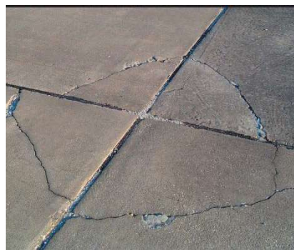
Figure C.11: PCC Corner Break.
