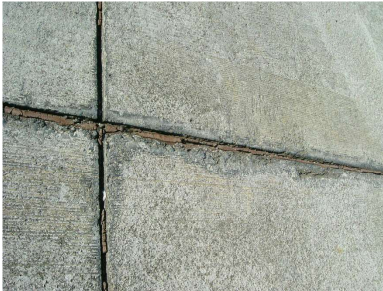
Figure C.13: PCC Joint Seal Damage.
