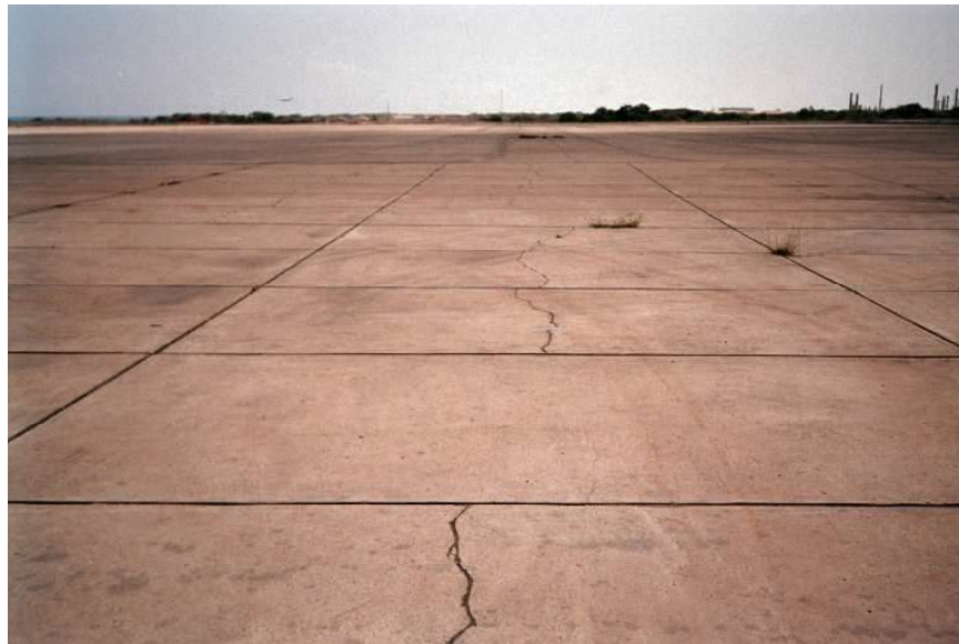
Figure C.12: PCC Transverse Cracks.
