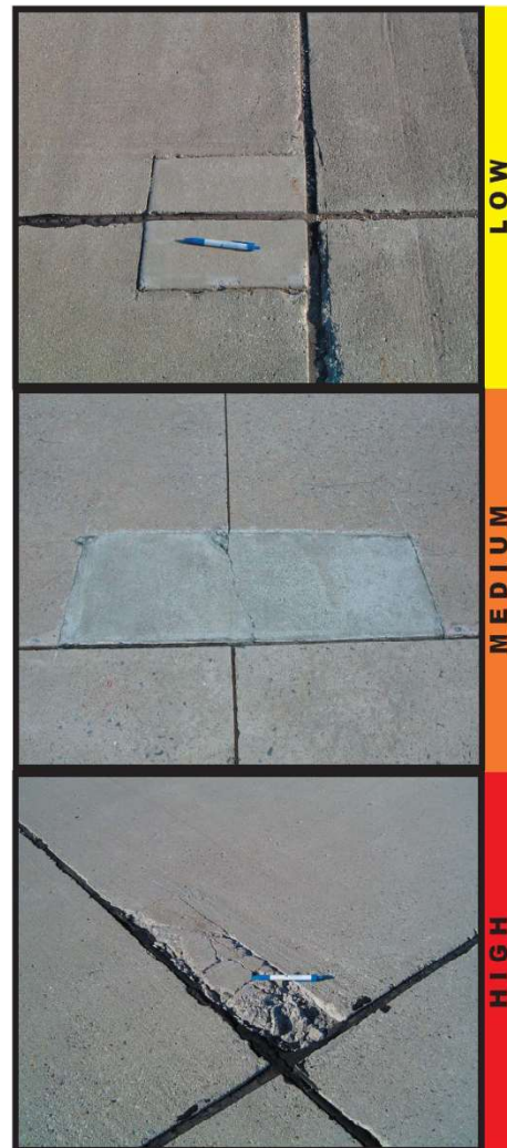
Figure C.14: PCC Small Patch.
