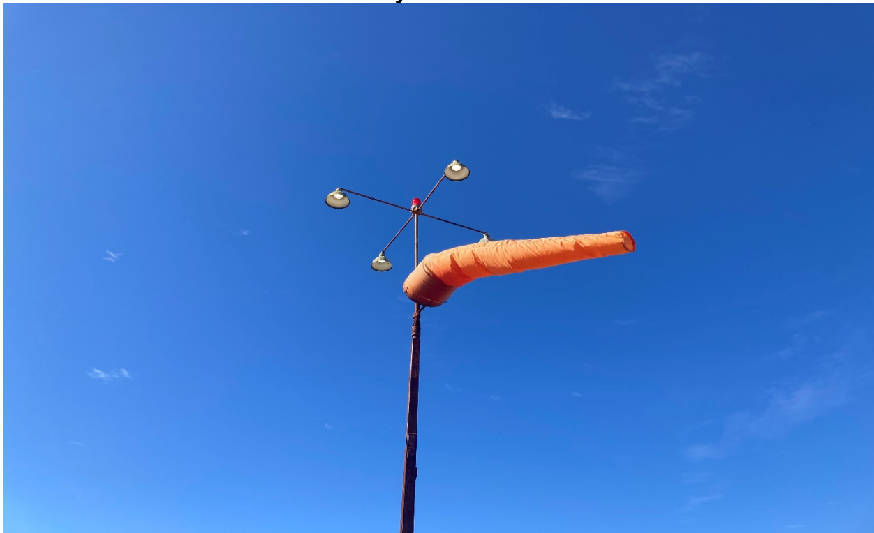
Photo #6 – Primary Wind Direction Indicator
