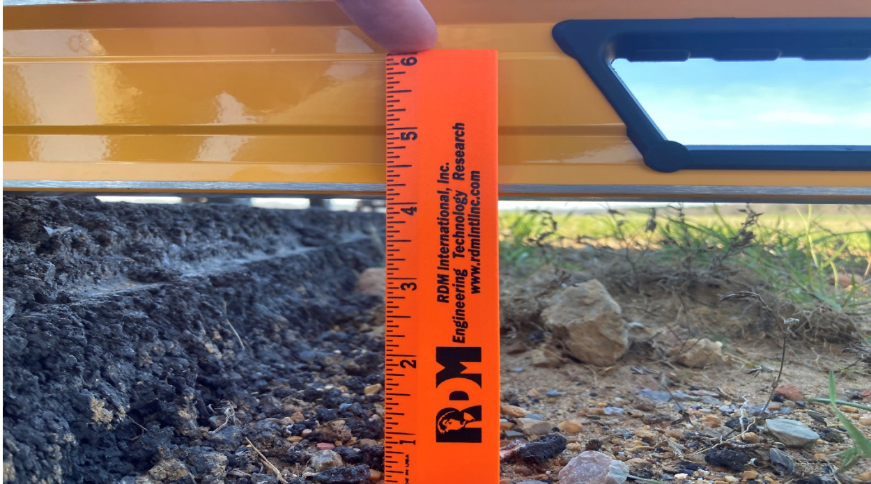
Photo #3 – Runway Edge Drop
