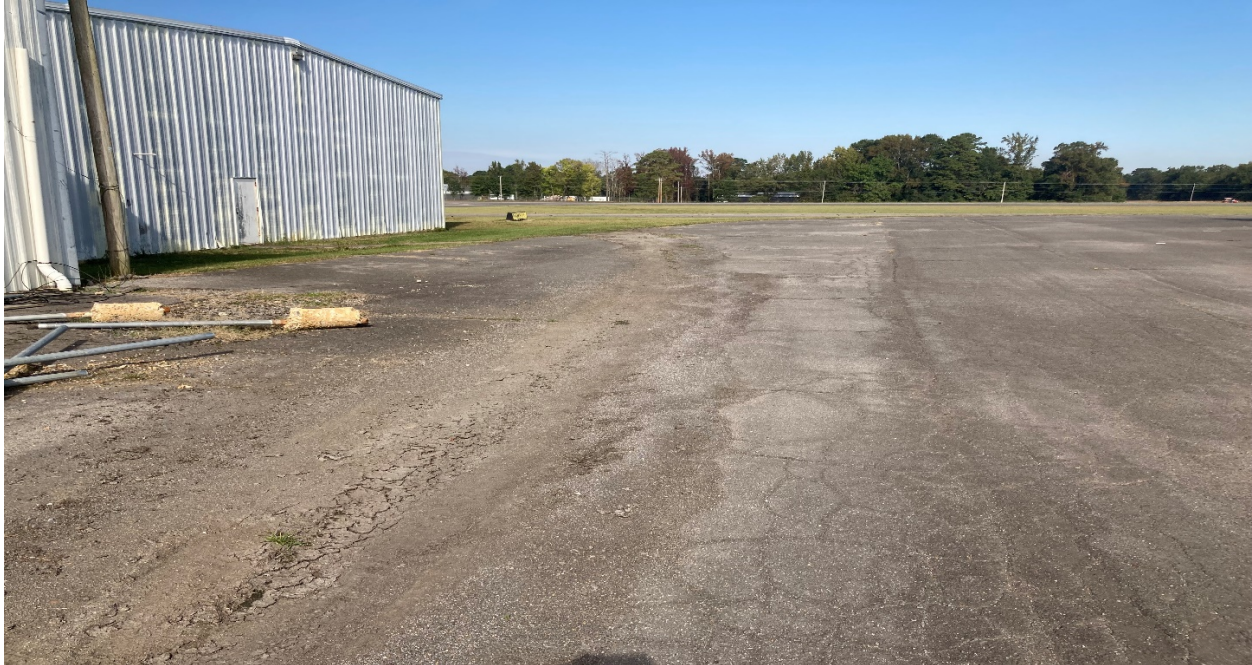
Photo #12 – Taxiway Pavement Failure
