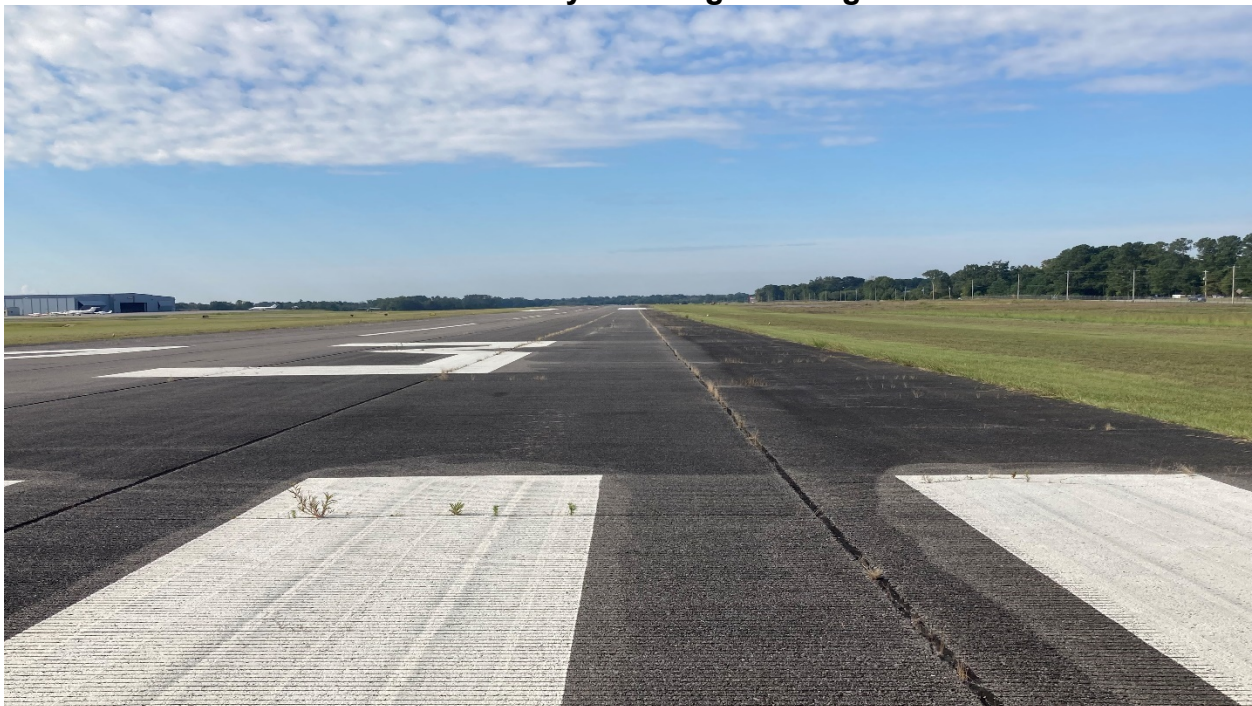
Photo #9 – Runway cracking with vegetation
