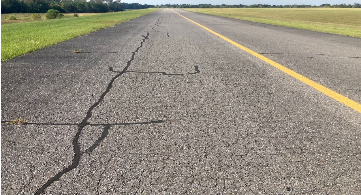
Photo #8 – Taxiway A Alligator Cracking
