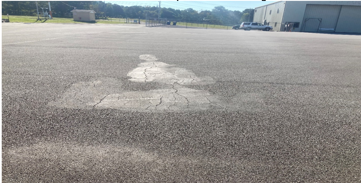
Photo #7 – Main Apron Patch Cracking
