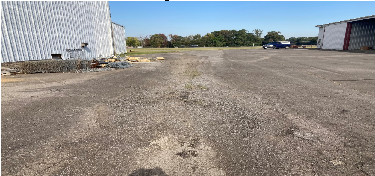
Photo #13 – Fencing Materials in Movement Area
