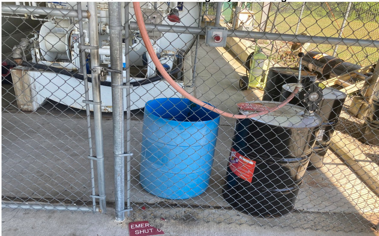
Photo #13 – Broken Emergency Shutoff Sign
