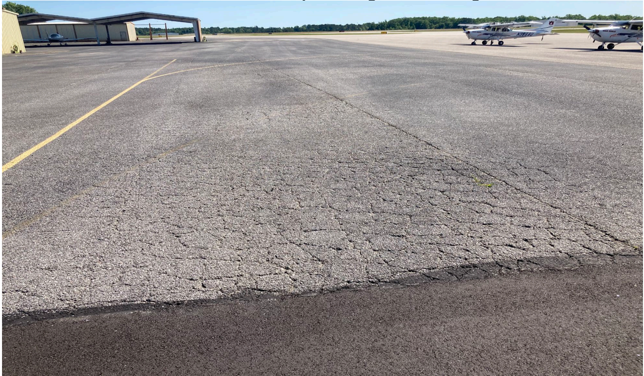
Photo #10 – West Apron Alligator Cracking
