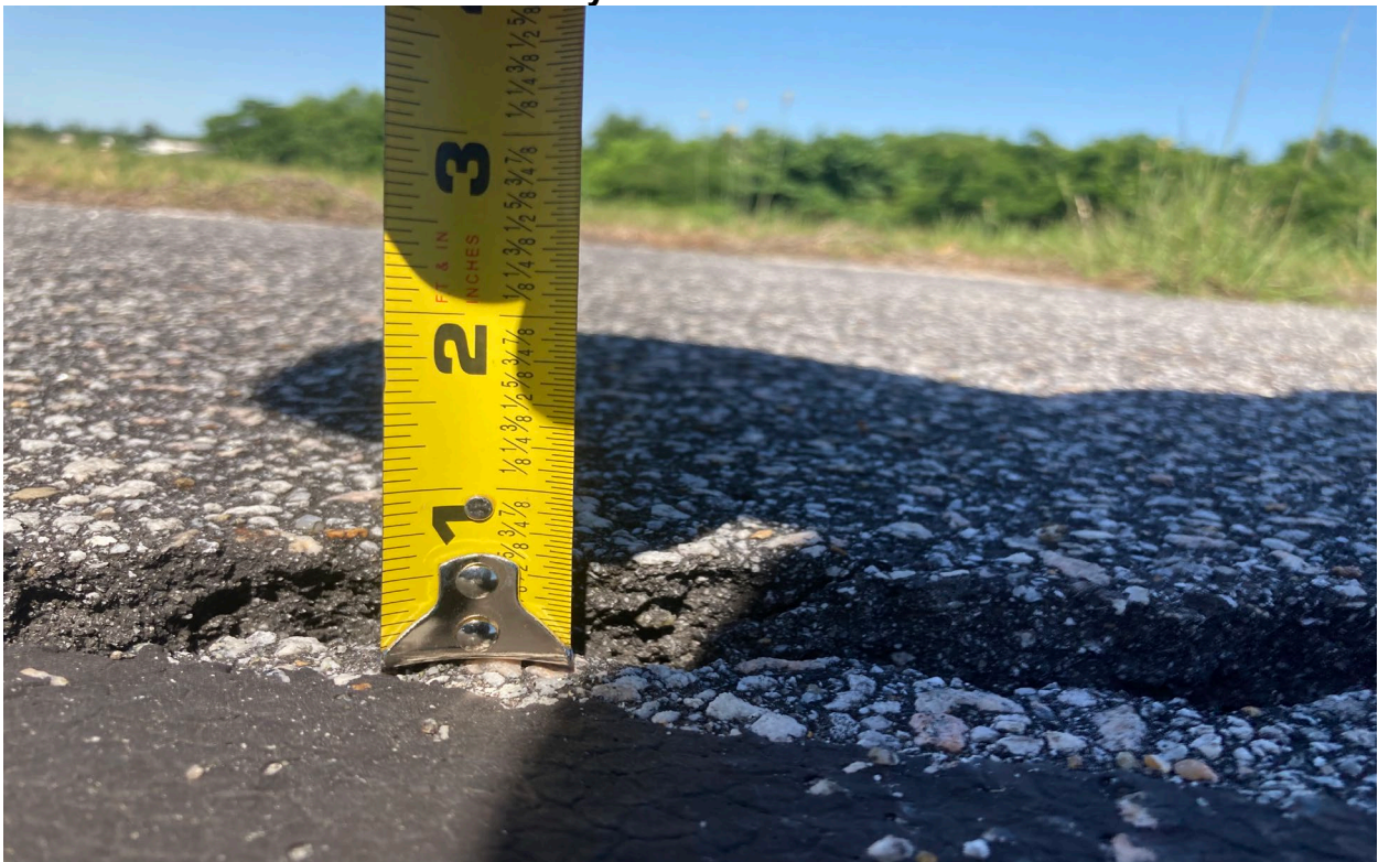
Photo #12 – Taxiway A Pavement Surface Variation
