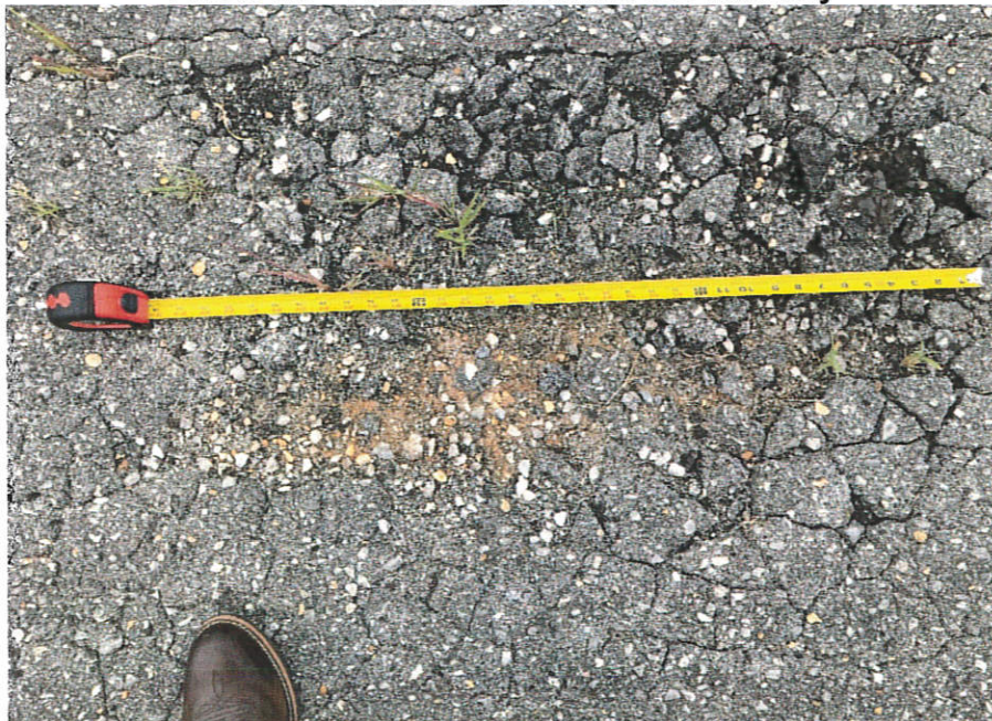
Photo #9– Pavement Failure on Taxiway
