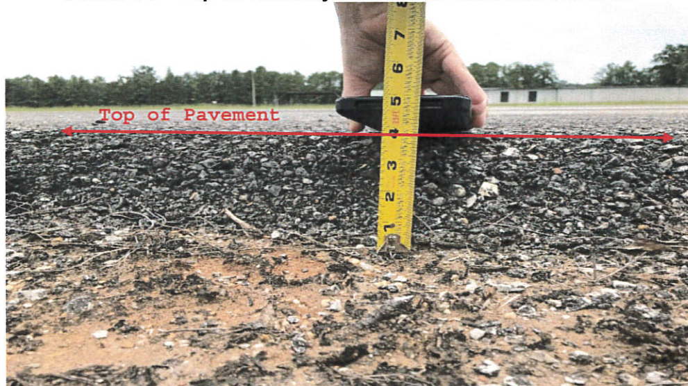
Photo #3 – Lip of Runway Pavement Exceeds 3 Inches
