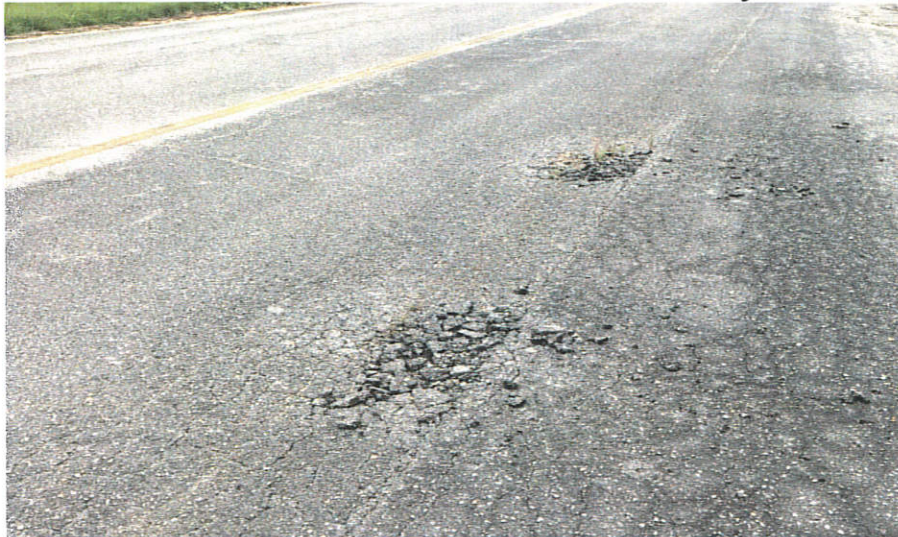
Photo #8– Pavement Failure on Taxiway
