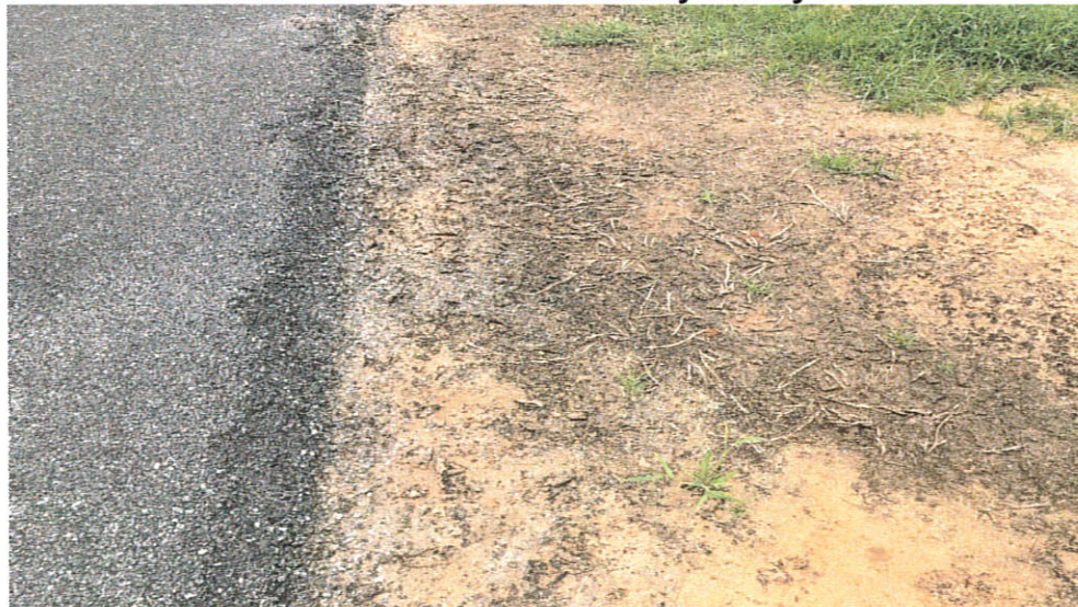
Photo #4 – Erosion in Runway Safety Area
