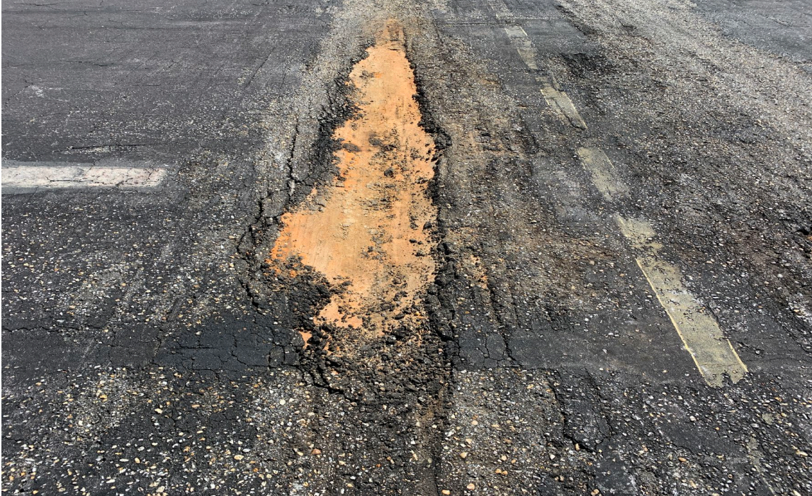
Photo # 8 – Severe Skid Damage (Failure) on Apron
