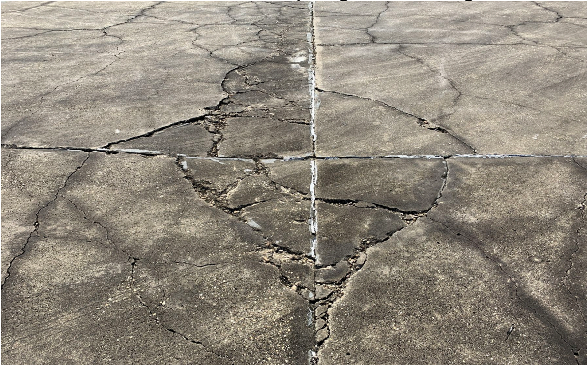
Photo # 11 – Severe Concrete Spalling and D-Cracking at Joint
