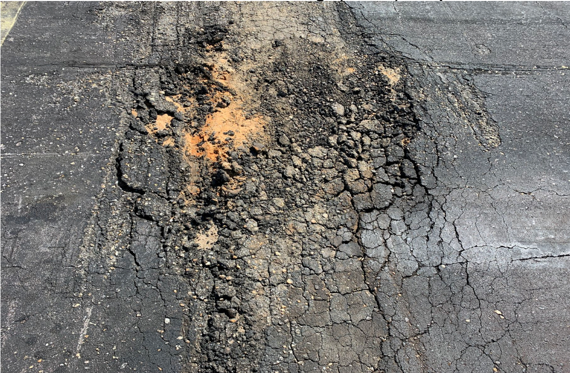
Photo # 9 – Severe Skid Damage (Failure) on Apron
