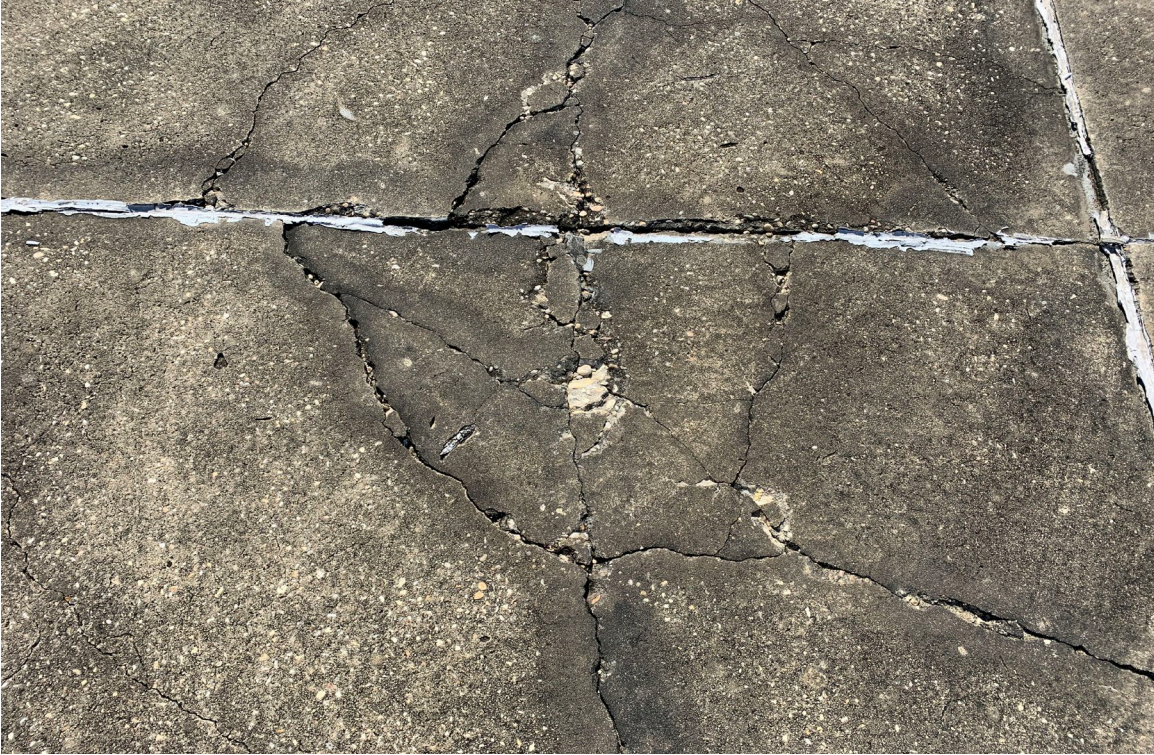
Photo # 12 – Concrete Spalling
