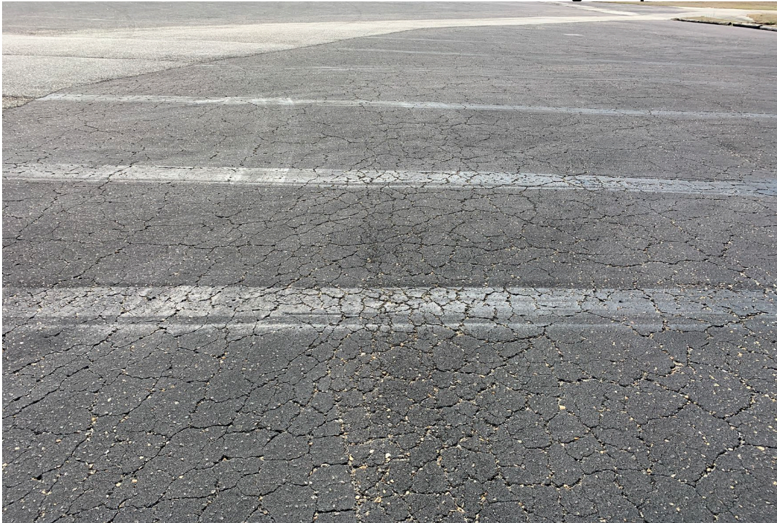
Photo # 7 — Extensive Micro-Surface Cracking on Apron
