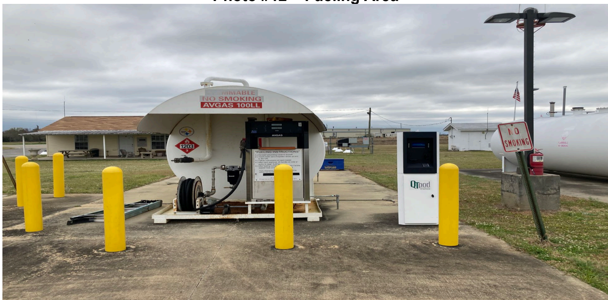
Photo #12 – Fueling Area
