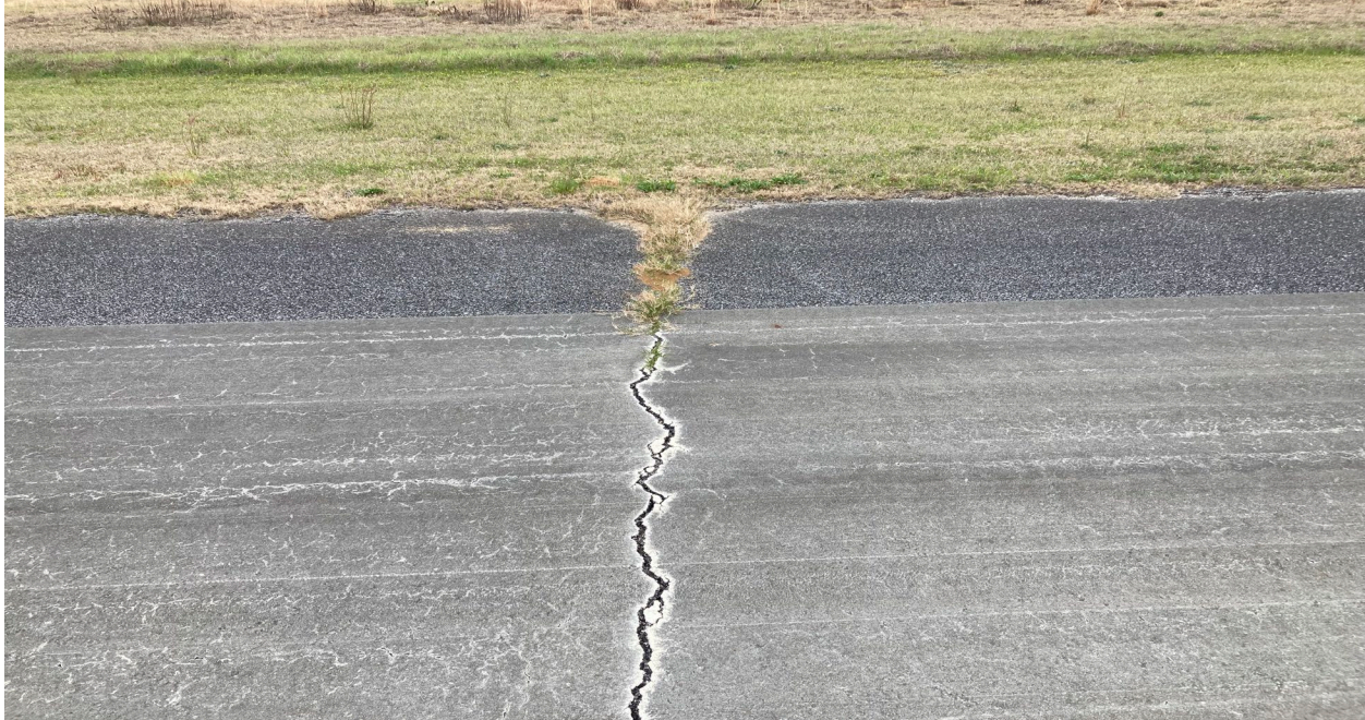
Photo #10 – Vegetation in Cracks on Runway
