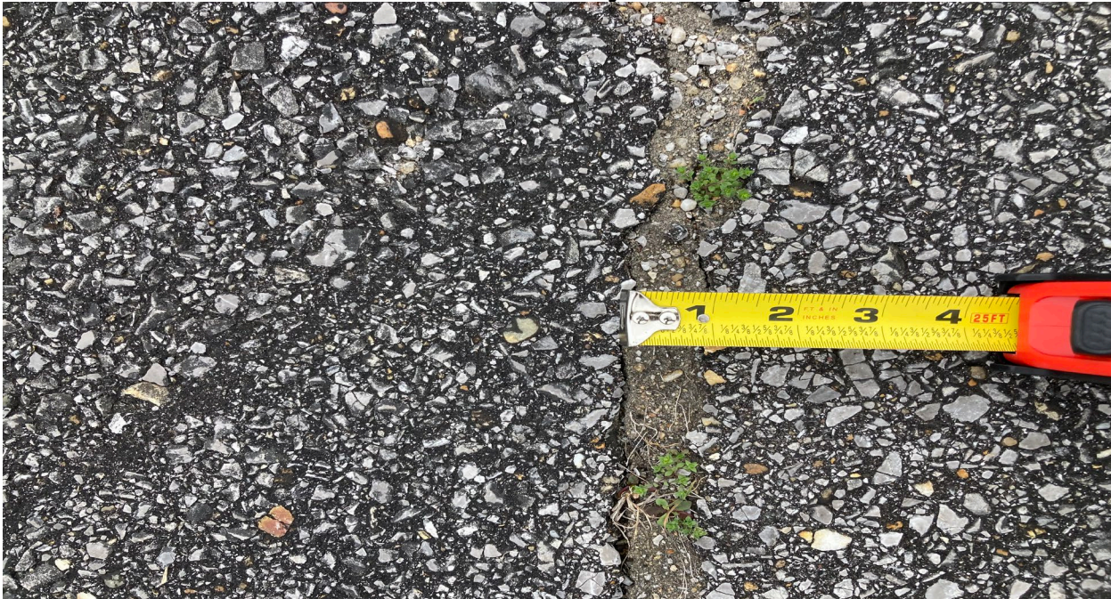
Photo #9 – Runway Cracking
