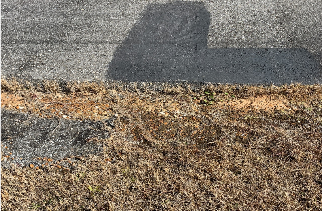
Photo # 4 – Erosion in Runway Safety Area
