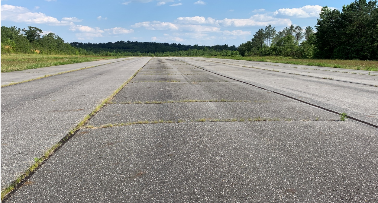
Photo # 9 – Block Cracking & Vegetation
