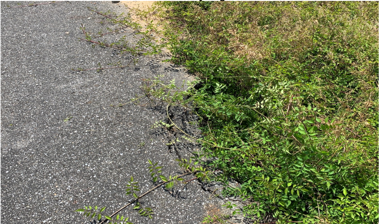
Photo #10 – Taxiway Edge Erosion
