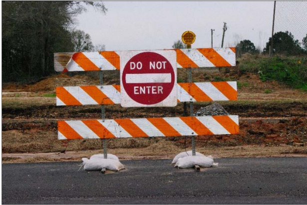
X Sheeting Peeling Off Top Rail
