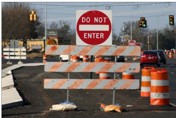
X Noticeably Faded Sheeting
