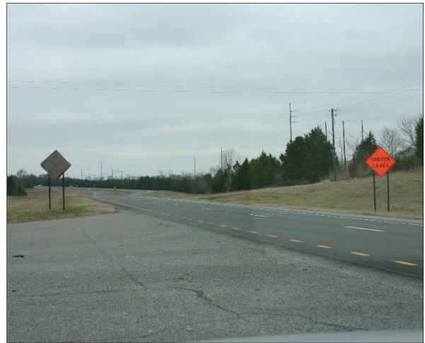
X Missing Sign Cover
