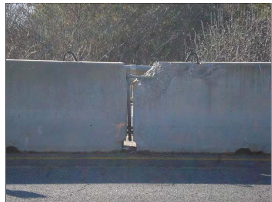
X Physical Damage
