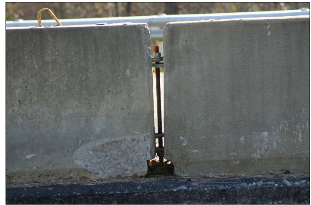
X Bolt Too Small (Minimum Diameter 1 1/4" Required)
