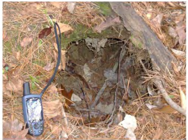
Roof collapse area in the southern part of the study area to the southeast of Alternate I
