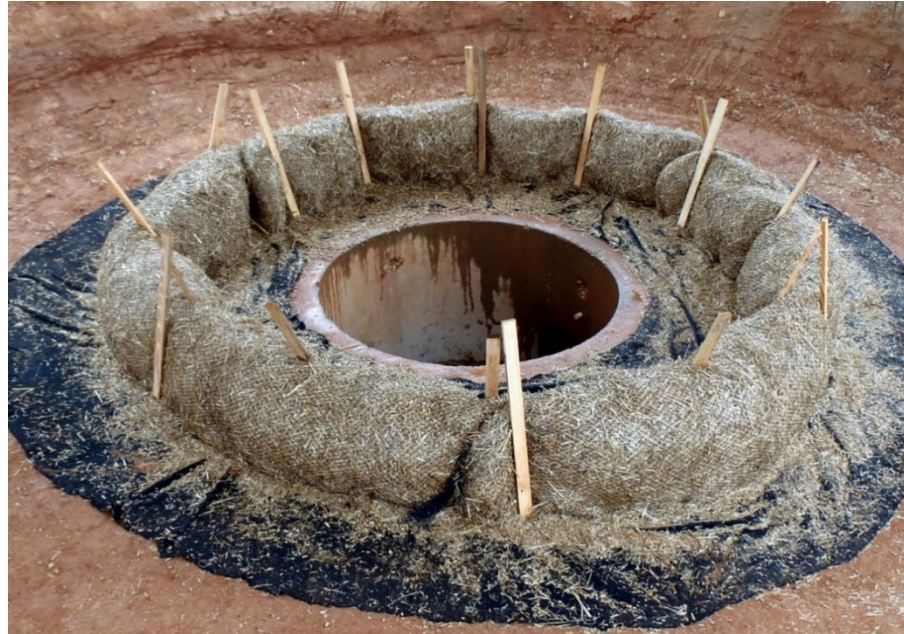
Figure IP-5 Wattle Inlet Protection Installation. (Photo courtesy of AU-SRF. See Appendix for CAD files)
