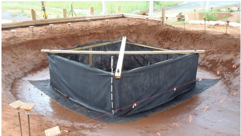
Figure IP-2 Silt Fence Inlet Protection Installation. (Showing silt fence, geotextile underlayment, steel T-posts, 2 x 4 bracing, and dewatering device.) (Photo courtesy of AU-SRF. See Appendix for CAD files)
