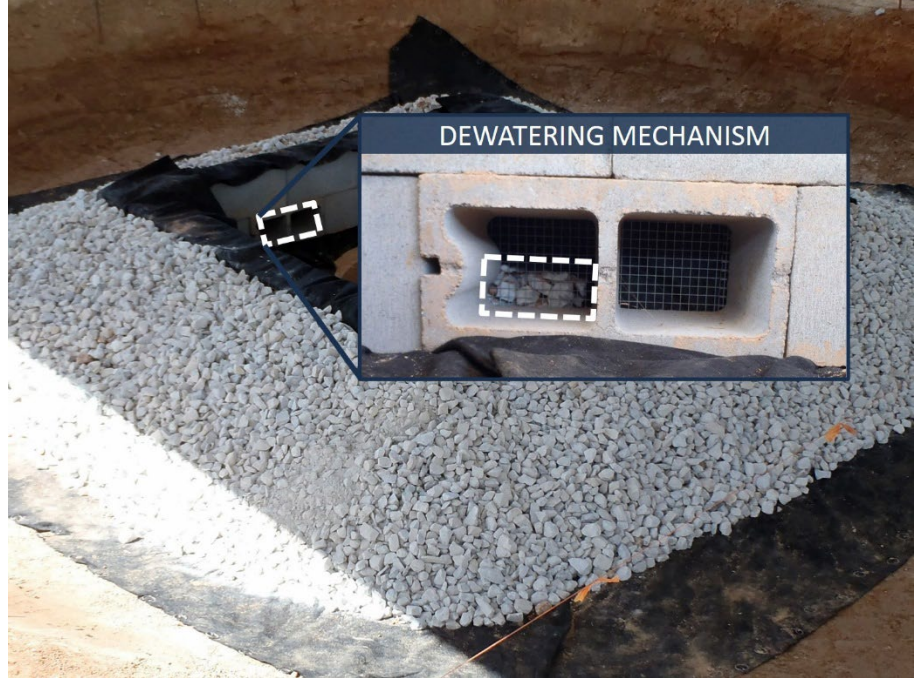
Figure IP-4 Block and Gravel Inlet Protection Installation. (Showing dewatering device.) (Photo courtesy of AU-SRF. See Appendix for CAD files)
