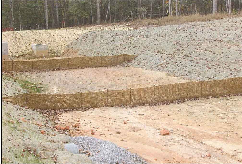
Figure SBN-2 Example of porous baffle made of 700 g/m 2 coir erosion blanket as viewed from the inlet.
