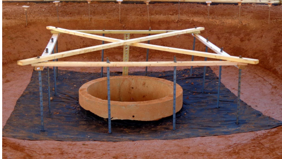
Figure IP-1 Silt Fence Inlet Protection Installation. (Showing geotextile underlayment, steel T-posts, 2 x 4 bracing, and dewatering device.) (Photo courtesy of AU-SRF. See Appendix for CAD files)
