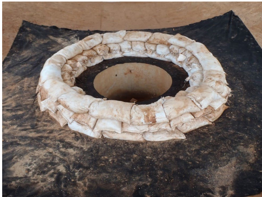
Figure IP-5 Sand Bag Inlet Protection Installation. (Photo courtesy of AU-SRF. See Appendix for CAD files)
