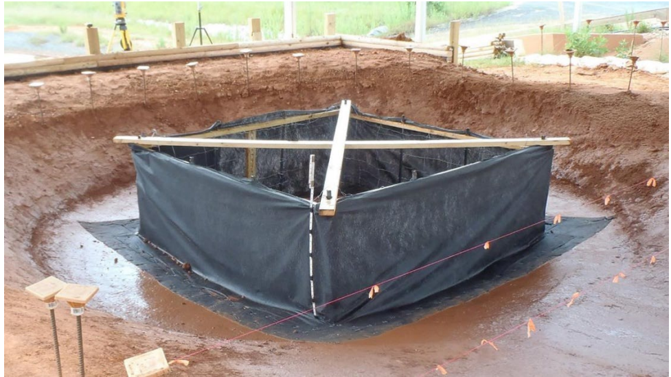
Figure IP-1 Silt Fence Inlet Protection Installation. (Showing silt fence, geotextile underlayment, steel T-posts, 2 x 4 bracing, and dewatering device.) (Photo courtesy of AU-SRF. See Appendix for CAD files)
