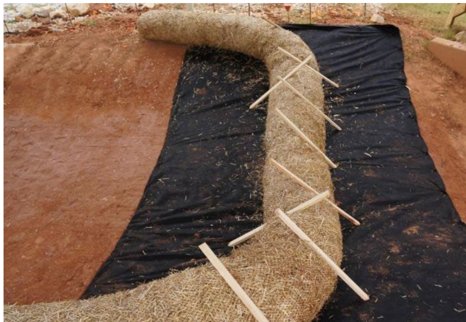
Figure CD-4 Wattle Check Dam (ditch check) (Photo courtesy of Auburn University Stormwater Research Facility)
