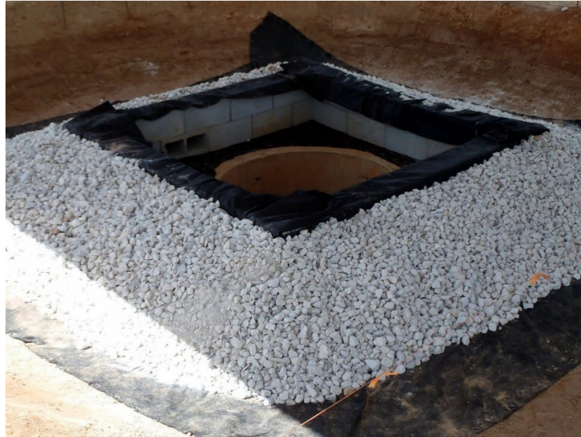
Figure IP-2 Block and Gravel Inlet Protection Installation. (Showing geotextile underlayment, gravel, and dewatering device.) (Photo courtesy of AU-SRF. See Appendix for CAD files)
