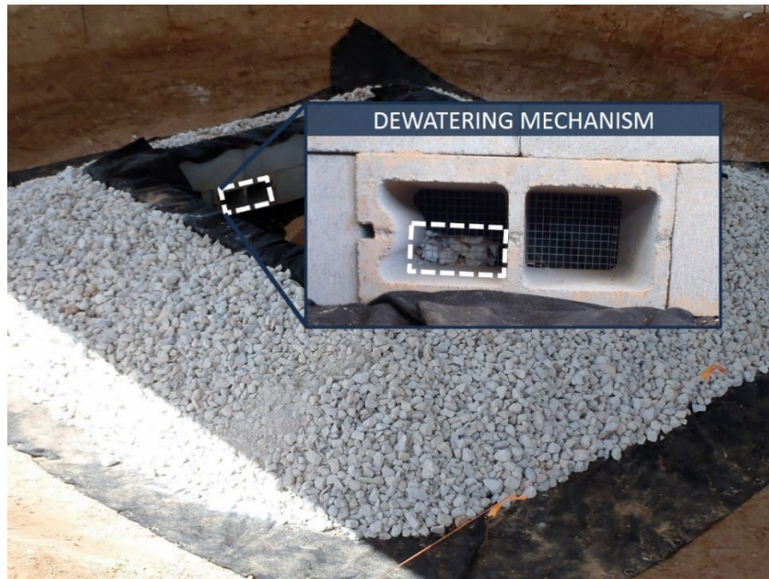
Figure IP-3 Block and Gravel Inlet Protection Installation. (Showing dewatering device.) (Photo courtesy of AU-SRF. See Appendix for CAD files)
