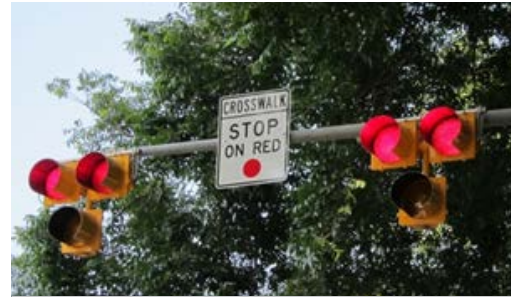
Example of PHBs mounted on a mast arm.
