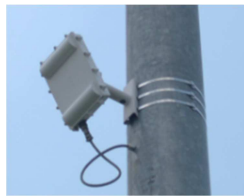
Figure 3. Pole-Mounted Radar Installation
