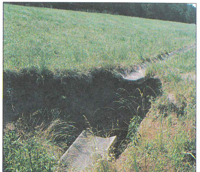
Displacement of Ditch Paving
