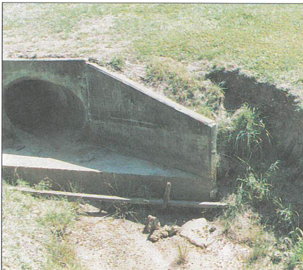
Scouring at Outlet
