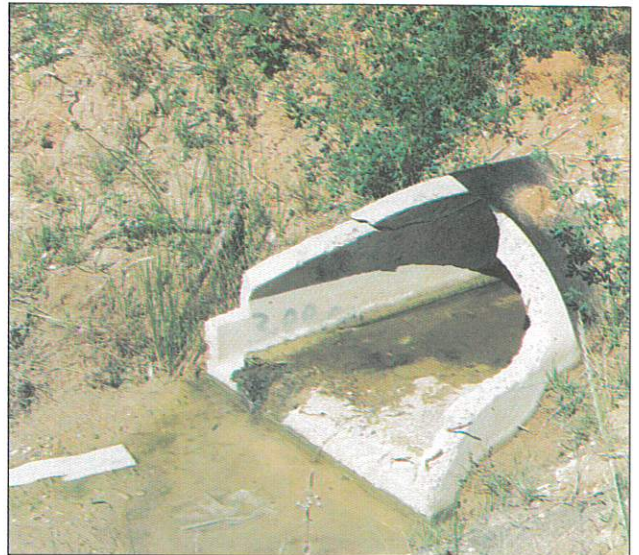
Damaged Pipe Culvert
