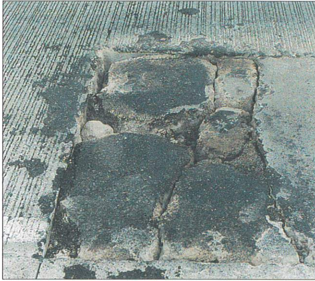
Concrete Pavement Failure
