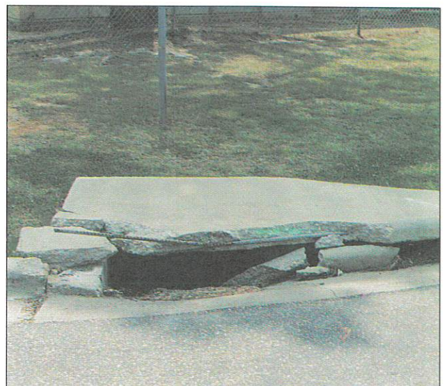
Damaged S-type Inlet
