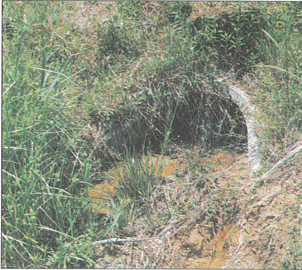
Blocked Pipe Culvert
