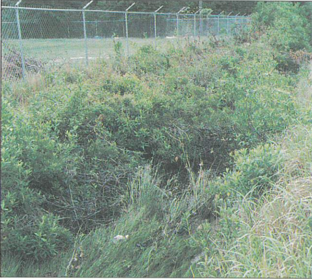
Vegetation Blocking Ditches
