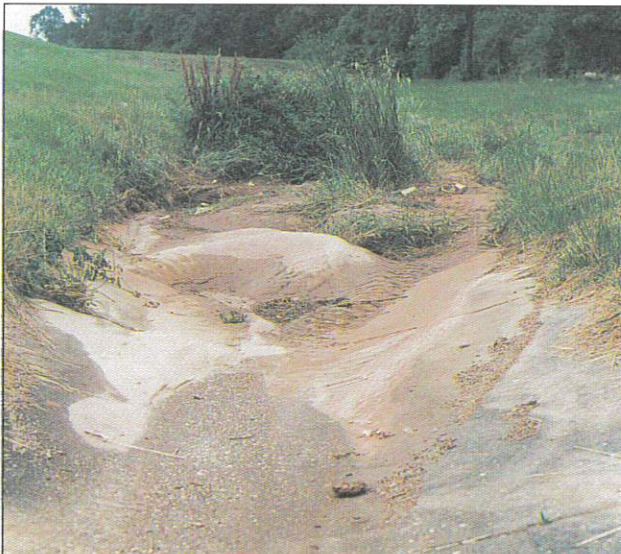
Siltation of Paved Ditch
