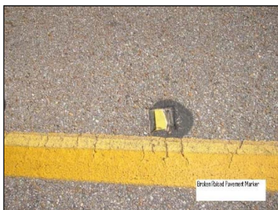
Damaged Raised Pavement Marker – Count as Deficient
