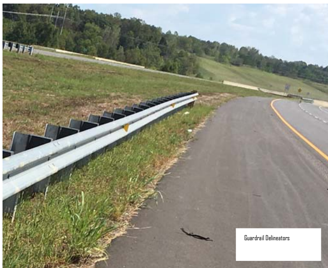
Functional Guardrail Delineator Do Not Count as Deficient
