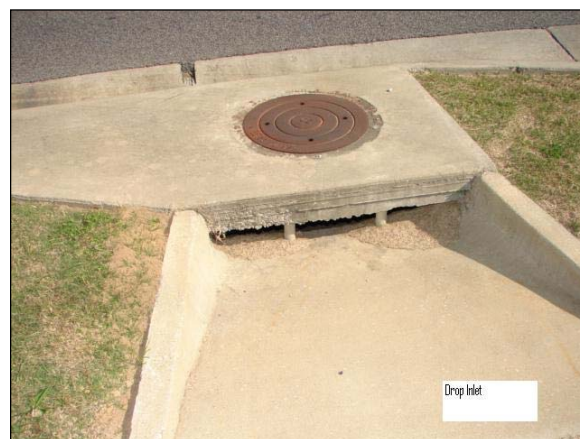
Deficient Drop Inlet Condition - Count as Deficient
