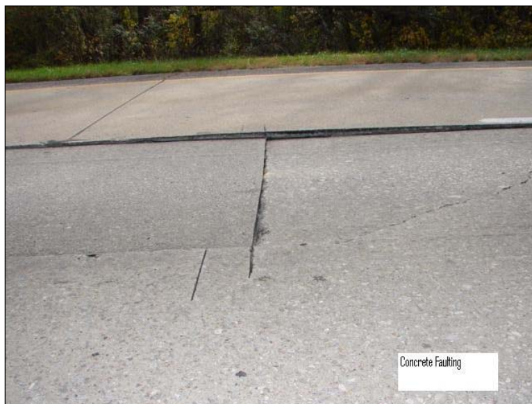
Sample Concrete Faulting
