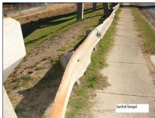
Deficient Guardrail Sample – Count Linear Feet of Deficiency
