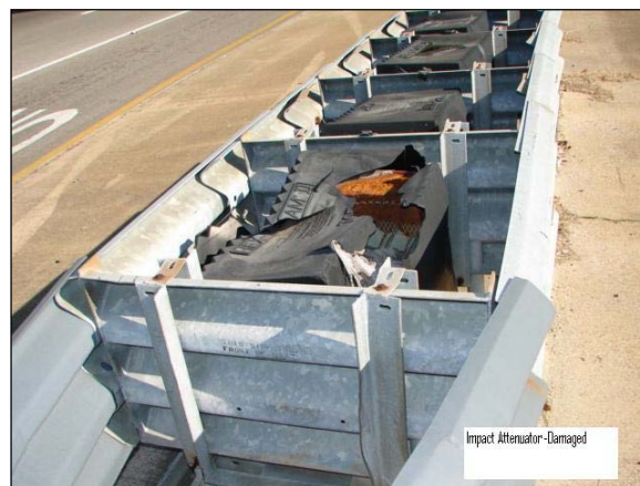
Deficient Impact Attenuator – Count as Deficient
