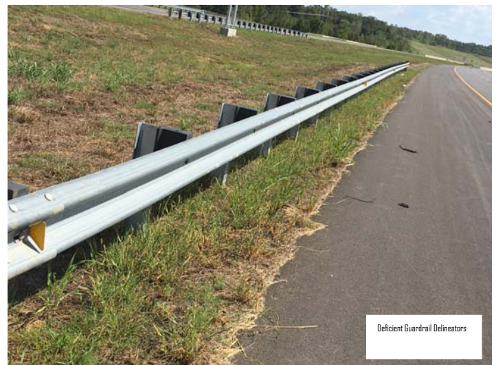
Deficient Guardrail Delineator (missing) Count as Deficient
