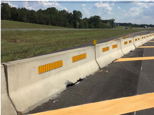
Functional Barrier Wall Delineator Do Not Count as Deficient
