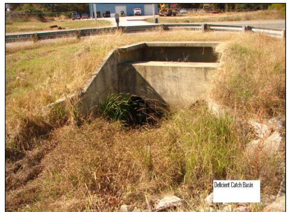
Deficient Catch Basin Condition - Count as Deficient
