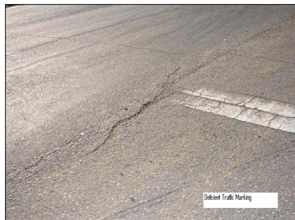
Deficient Pavement Marking Sample – Count as Deficient
