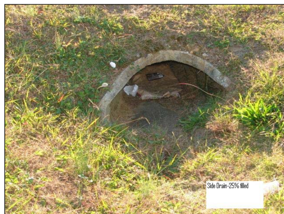
Deficient Side Drain Condition - Count as Deficient
