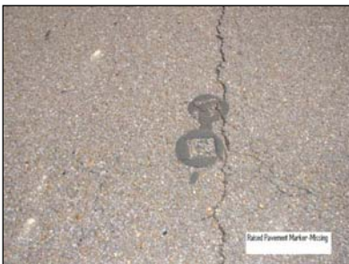
Missing Raised Pavement Marker – Count as Deficient
