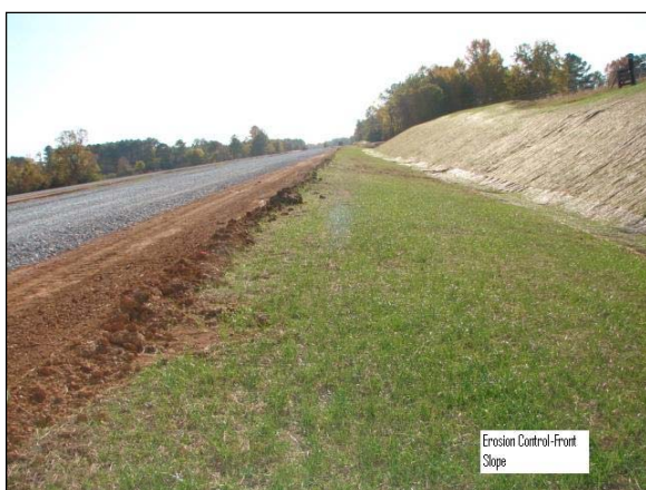
Functional Front Slope Condition - Do Not Count as Deficient
