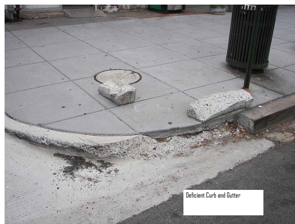
Deficient Curb and Gutter Condition - Count Linear Feet of Deficiency
