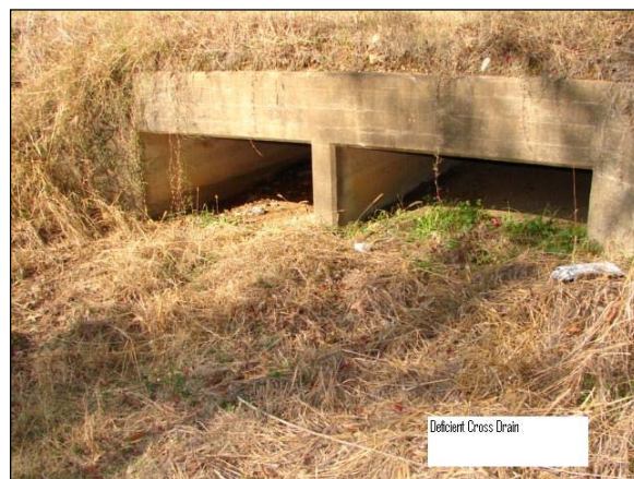
Deficient Cross Drain Condition - Count as Deficient
