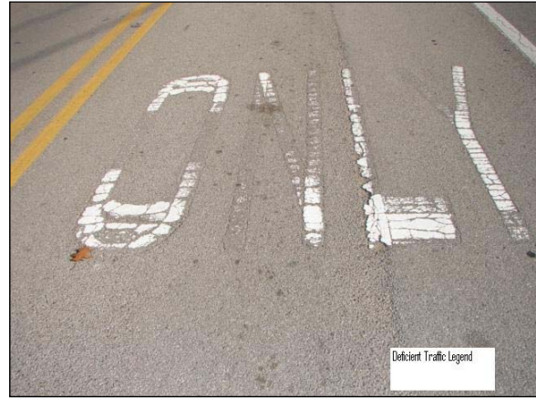
Deficient Pavement Legend Sample – Count as Deficient
