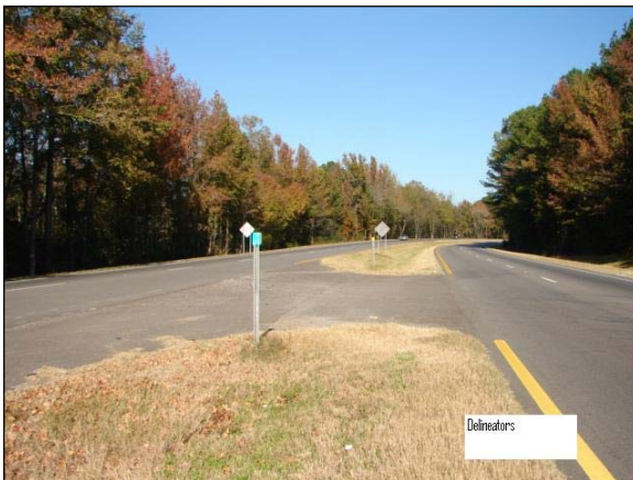
Functional Delineator – Do Not Count as Deficient
