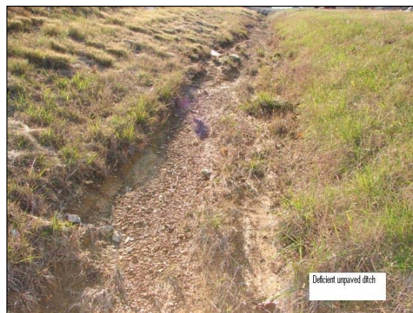
Deficient Unpaved Ditch Condition - Count Linear Feet of Deficiency
