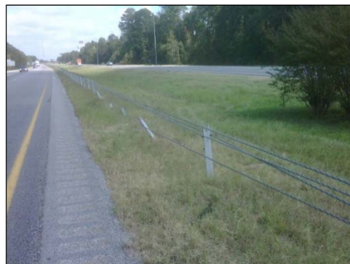
Deficient Cable Rail Sample – Count Linear Feet of Deficiency
