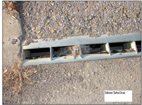
Deficient Slotted Drain Condition - Count as Deficient
