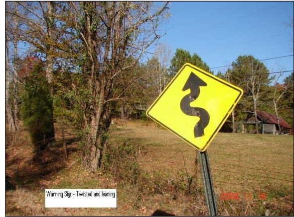
Deficient “Warning Sign” Sample – Count as Deficient
