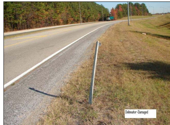
Deficient Delineator – Count as Deficient
