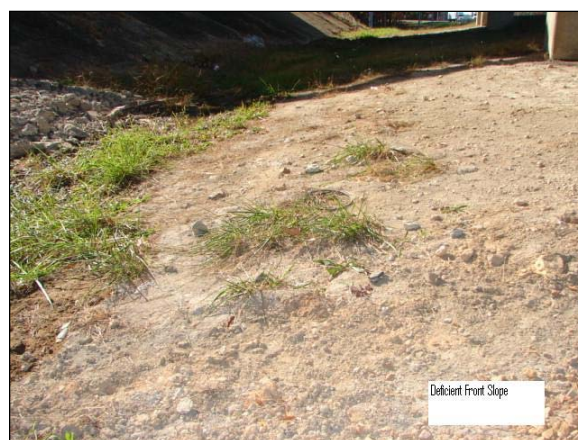
Deficient Front Slope Condition - Count Linear Feet of Deficiency
