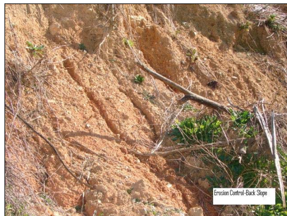
Deficient Back Slope Condition - Count Linear Feet of Deficiency
