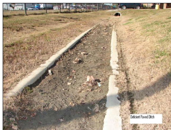
Deficient Paved Ditch Condition - Count Linear Feet of Deficiency
