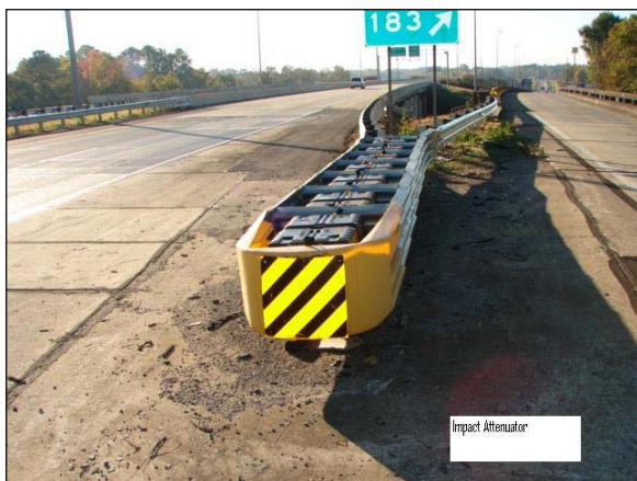
Functional Impact Attenuator – Do Not Count as Deficient
