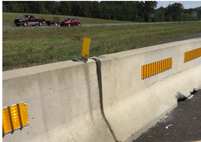
Deficient Barrier Wall Delineator (damaged) Count as Deficient
