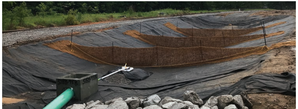
A sediment control basin which is a part of the storm water management at SR-158 extension project from Lott Road to Schillinger Road.
