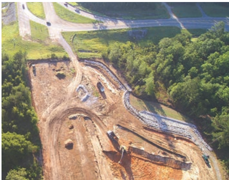
An aerial view of the SR-158 extension project from Lott Road to Schillinger Road.
