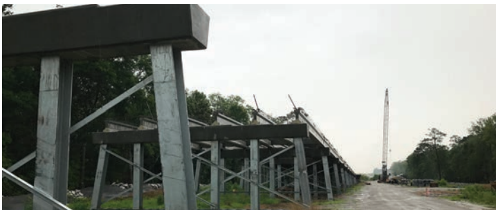
Eastbound bridge extension over Big Creek. ALDOT is prepping the super structure and setting girders.
