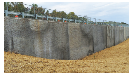
top Cherokee County landslide above SR-9
