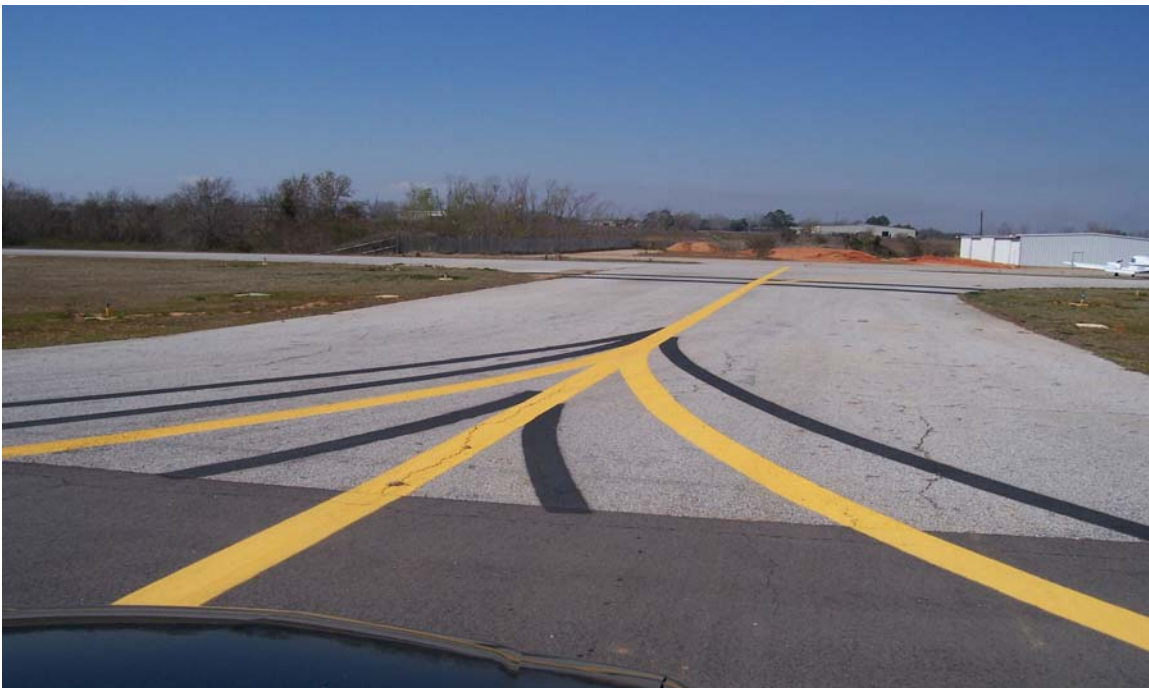
Photo # 2 – Painted Over Markings
