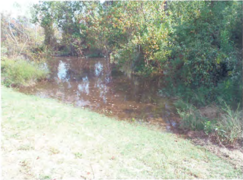
(42) Floodgate clogged with debris.
