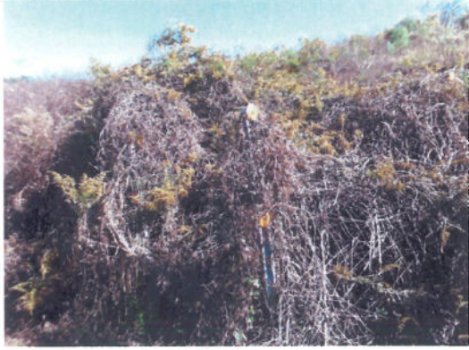
(27) Junction Box covered with vegetation
