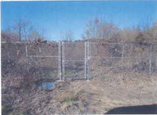
(16) Lock on gate on southern side of Lower Kilby Ditch off Northern Blvd. has been replaced and is now inaccessible.
