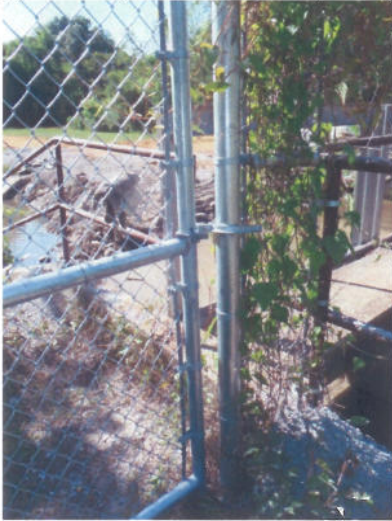
(3) Illegal dumping within fence indicates unauthorized entry
