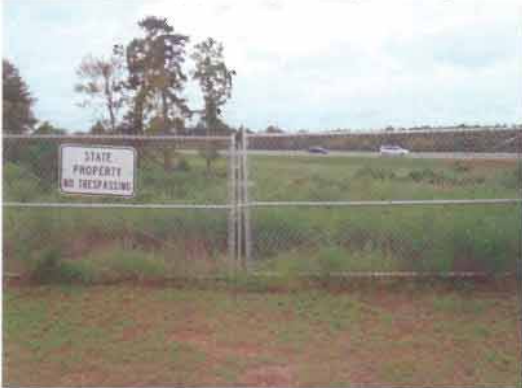
(3) Entry gate for upper Kilby Ditch by landscape berm is not operational.
