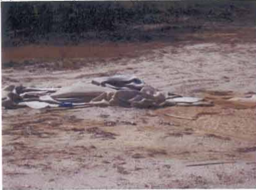
(5) Erosion to road
