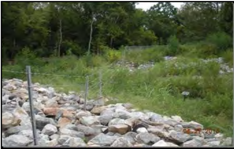
Outlet protection at Lower Kilby Ditch flow into Three Mile Branch; post-construction.
