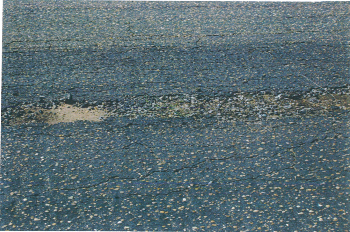
Photo # 7 – Runway with Pothole and Debris
