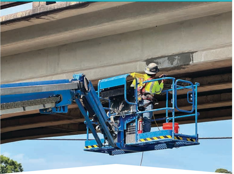
The region worked quickly to address and repair damage to the Wrights Mill Road bridge over I-85 North following a crash.
