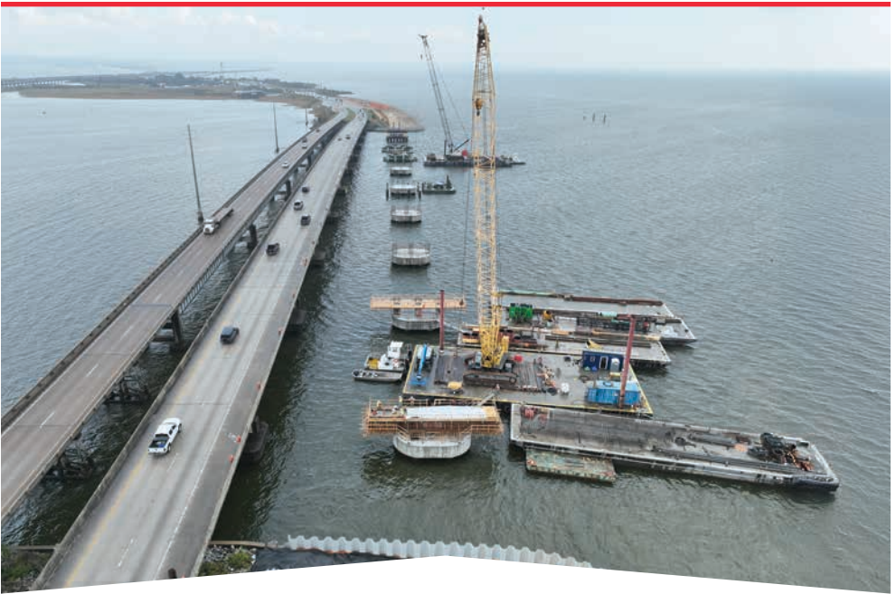
The Tensaw River Bridge Replacement Project is underway. The finished bridge will improve traffic and connectivity for drivers, pedestrians, and cyclists.
