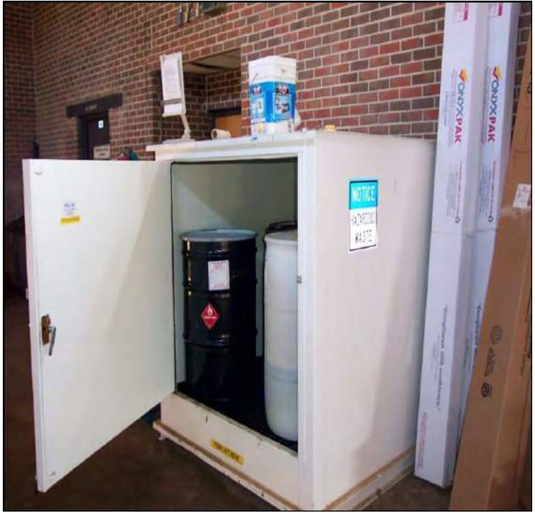
Hazardous Material Isolation
