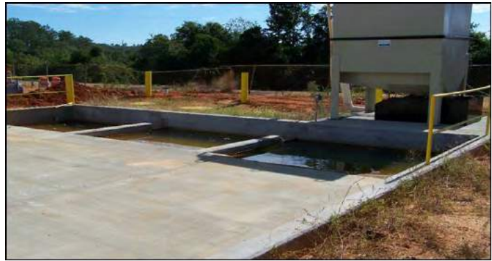
Wash Water Control
