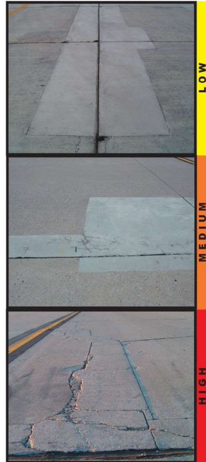
Figure C.15: PCC Large Patch.
