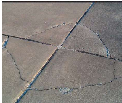
Figure C.11: PCC Corner Break
