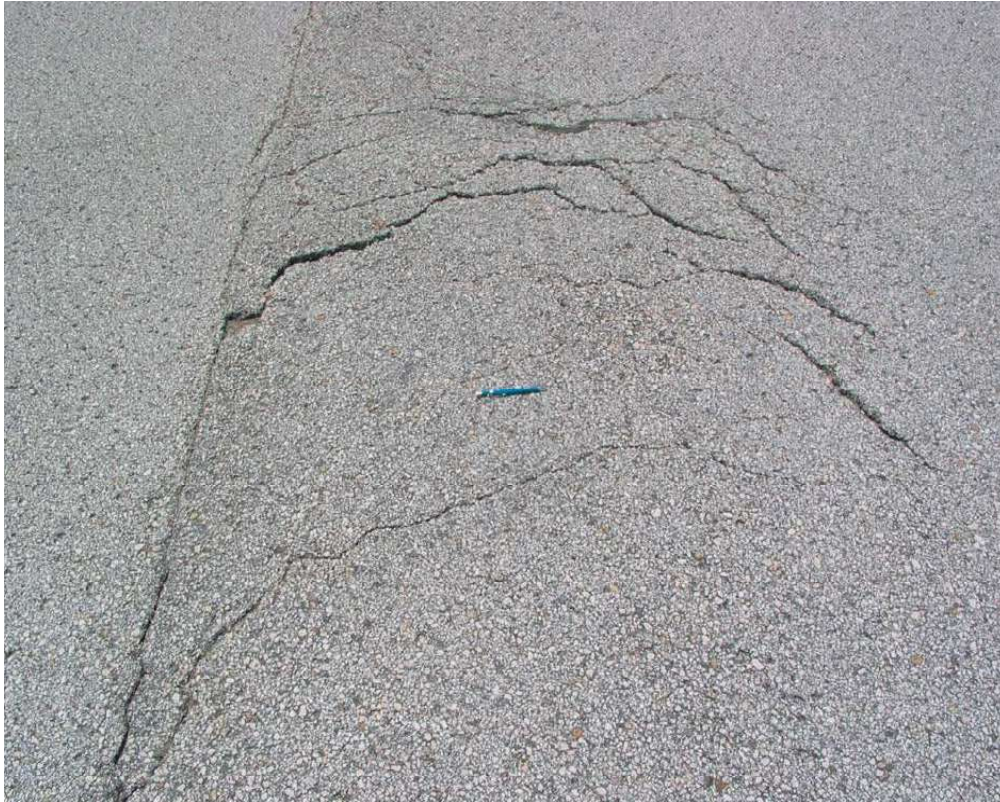
Figure 14-1. Slippage Cracking in Asphalt Concrete
