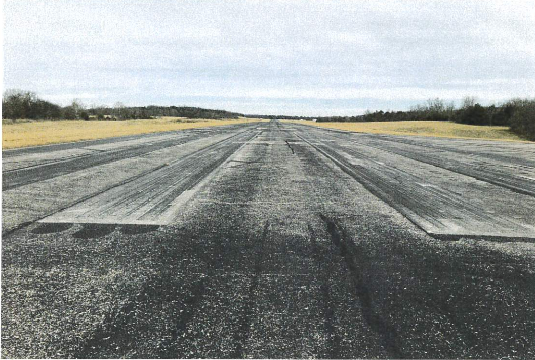
Photo #6 – NP Markings Runway 2
