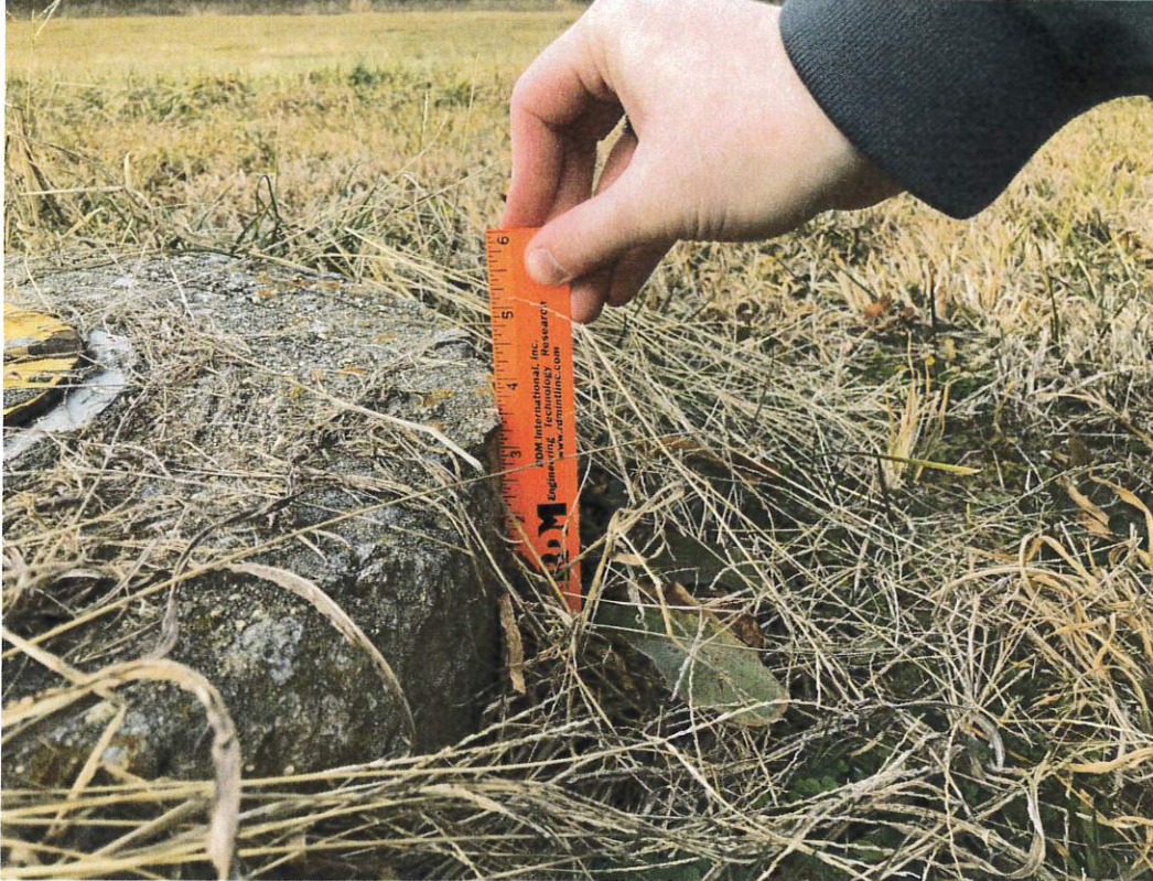
Photo #5— Runway Light Base
