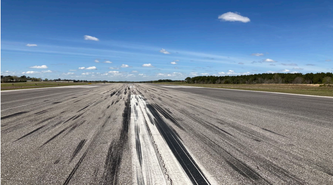
Photo #4-Runway 29 Rubber Accumulation
