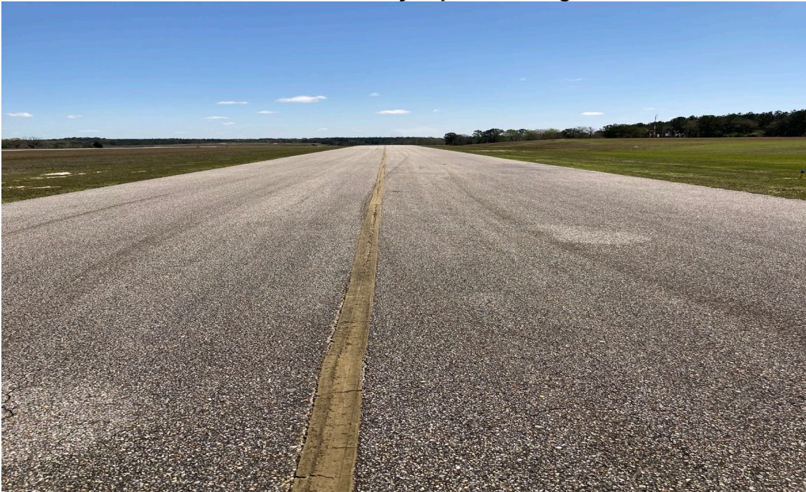
Photo #5-Taxiway Alpha Markings
