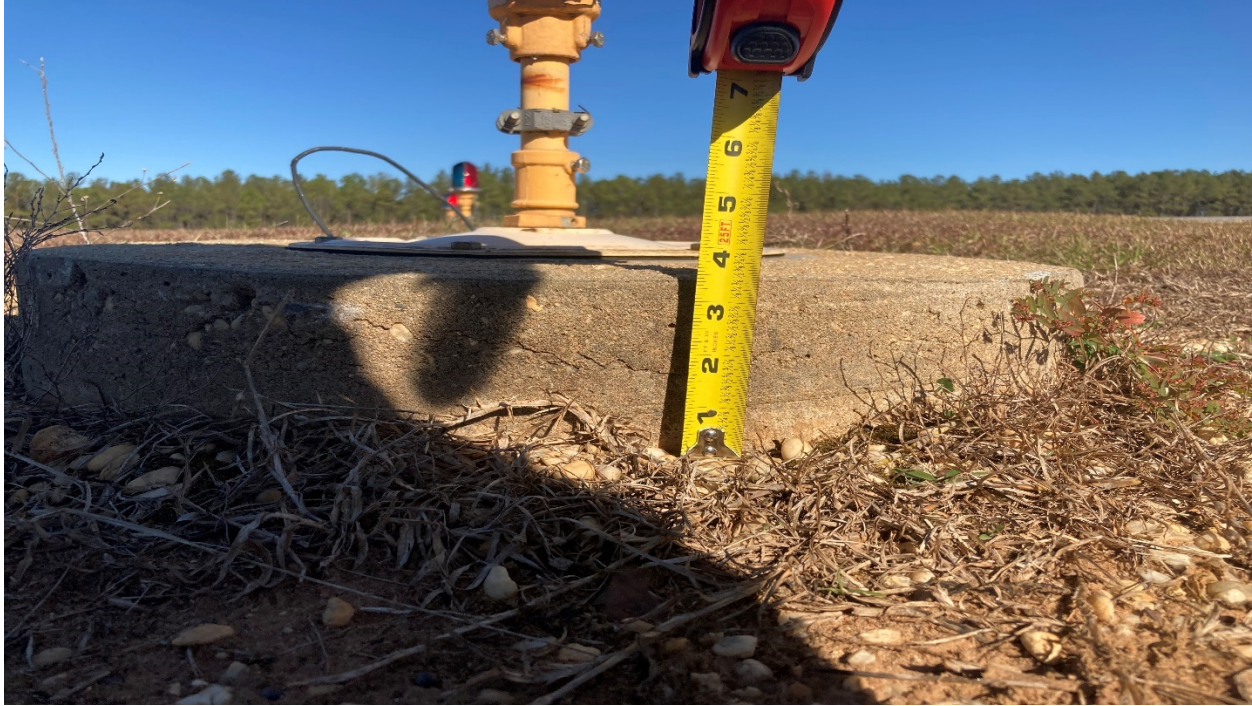
Photo #4 – Runway 8 Threshold Light Base
