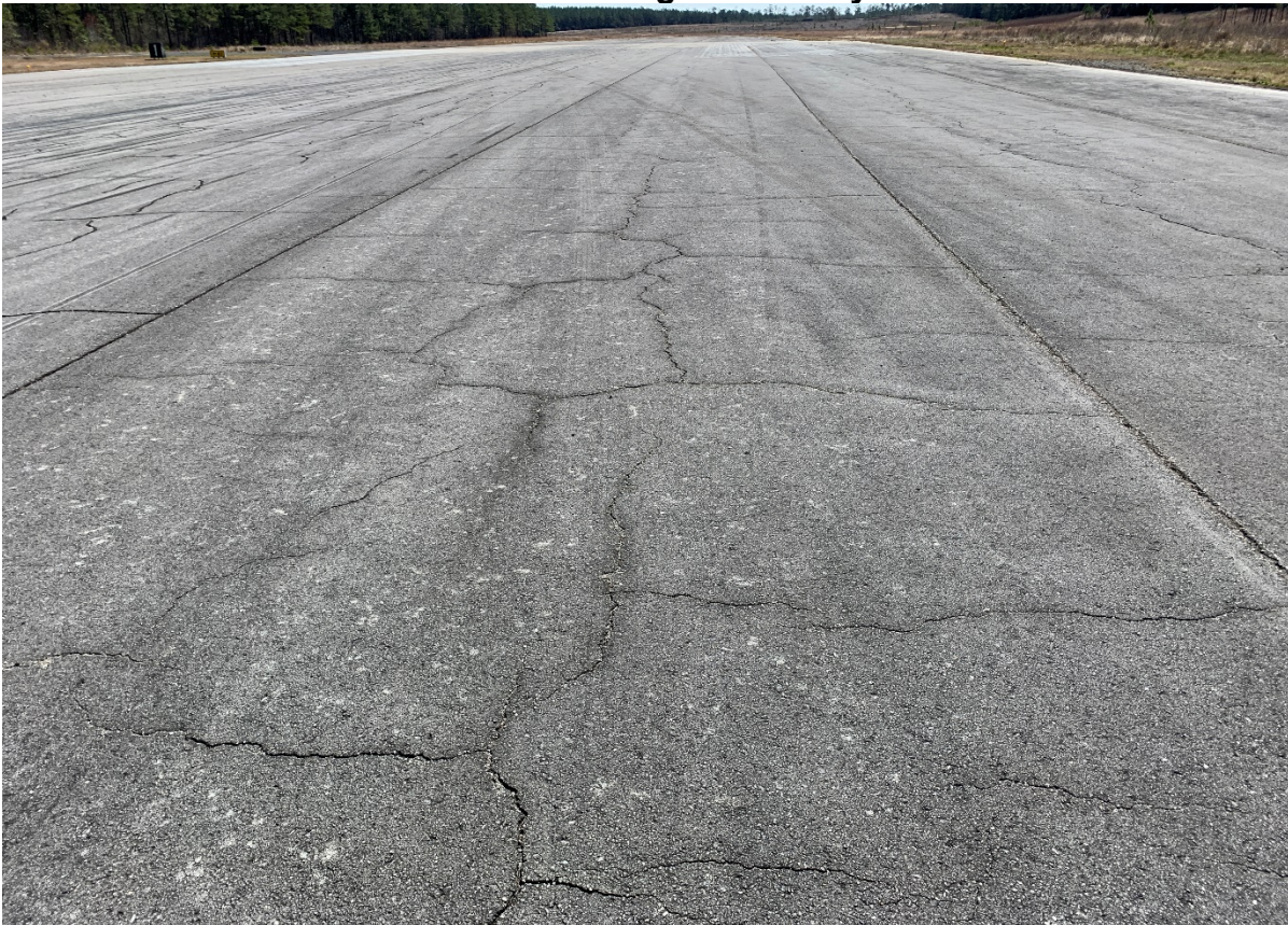
Photo #11—Cracking on Runway 12/30
