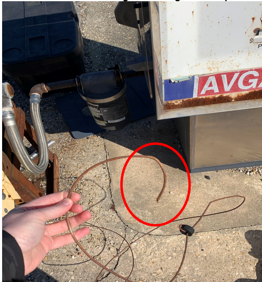
Photo #13—Missing Grounding Cable Clip
