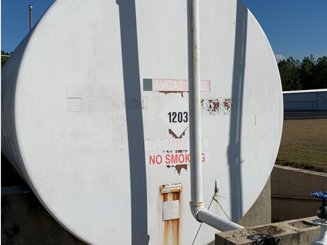
Photo #14 – Fuel Tank Contents Label Faded
