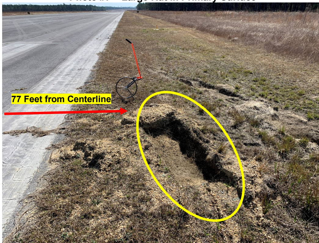
Photo #7 – Large Rut in Primary Surface
