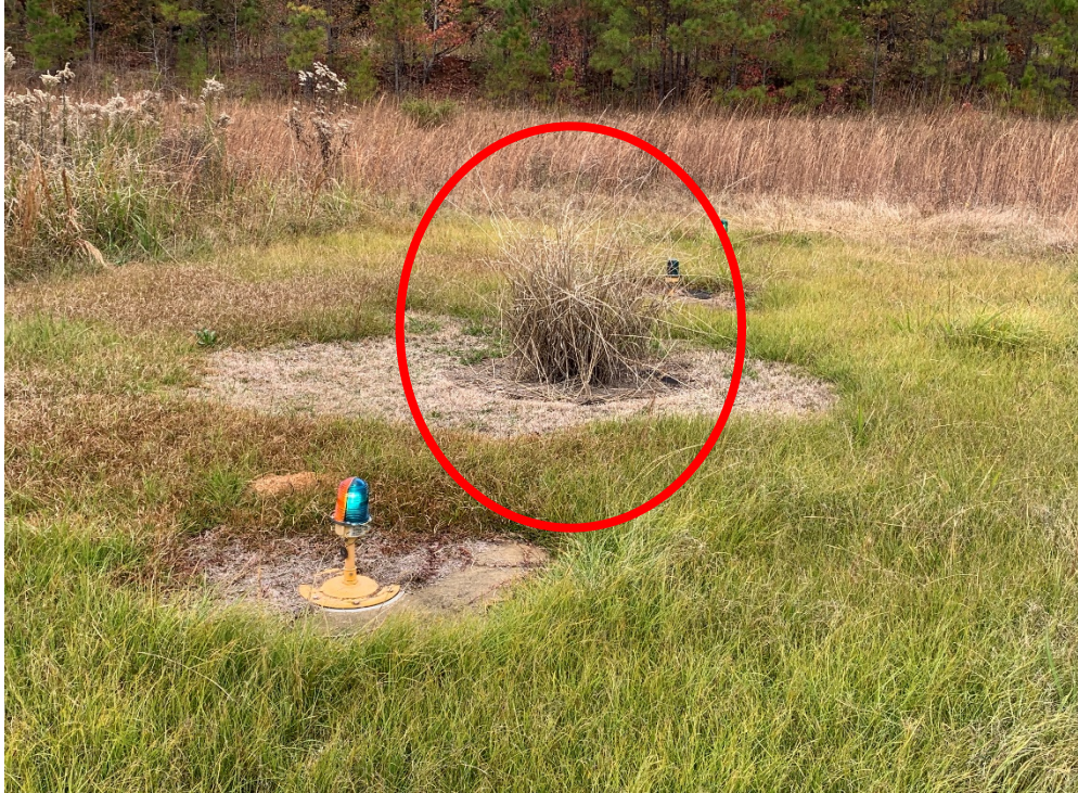
Photo #10 – Runway Threshold Light Obscured
