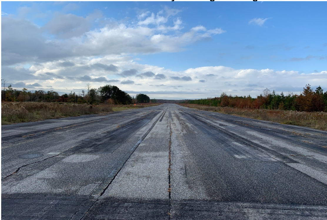
Photo #6 – NPI Runway Markings Missing
