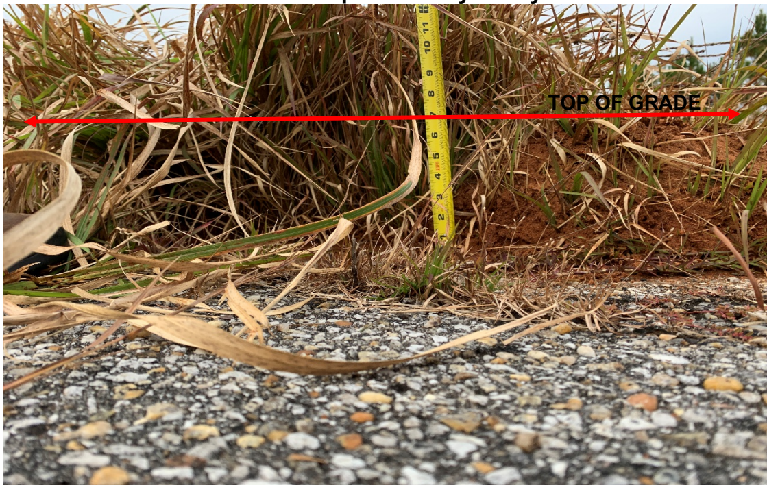
Photo #5 – Hump in Runway Safety Area
