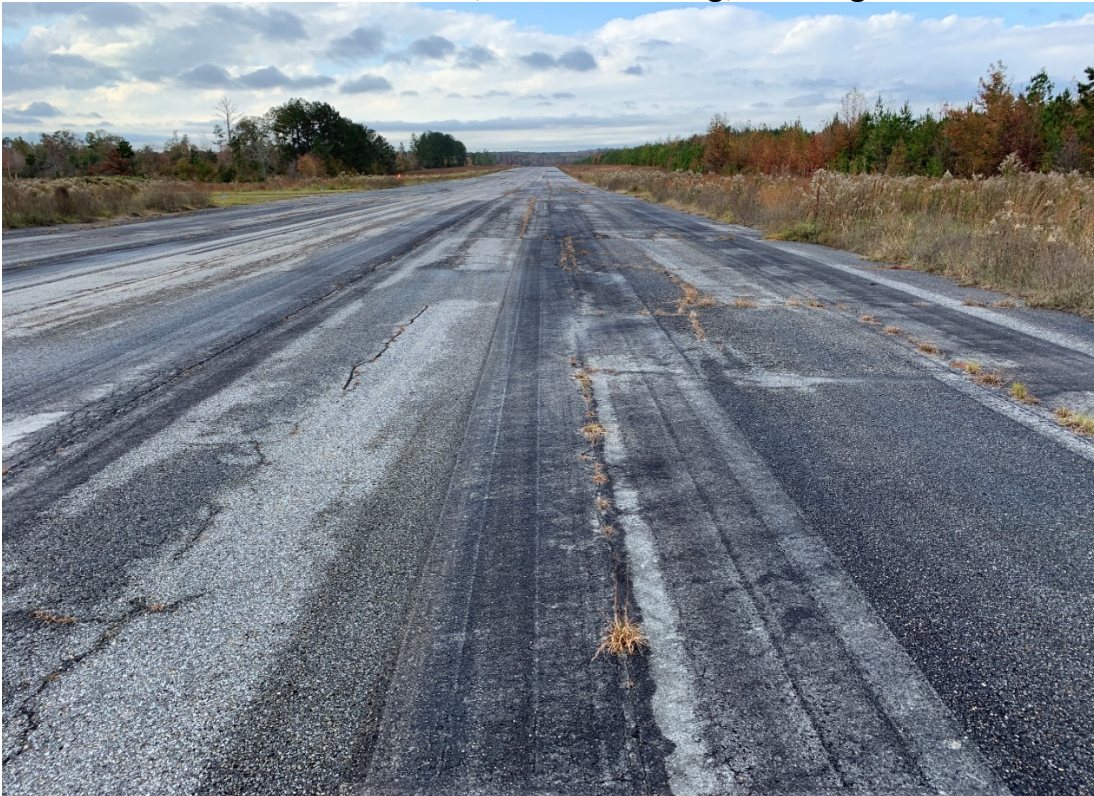
Photo #11 – Crack Seal Failure, Block Cracking, and Vegetation Growth
