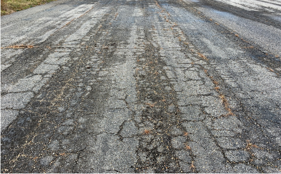
Photo #12 – Alligator Cracking on Runway
