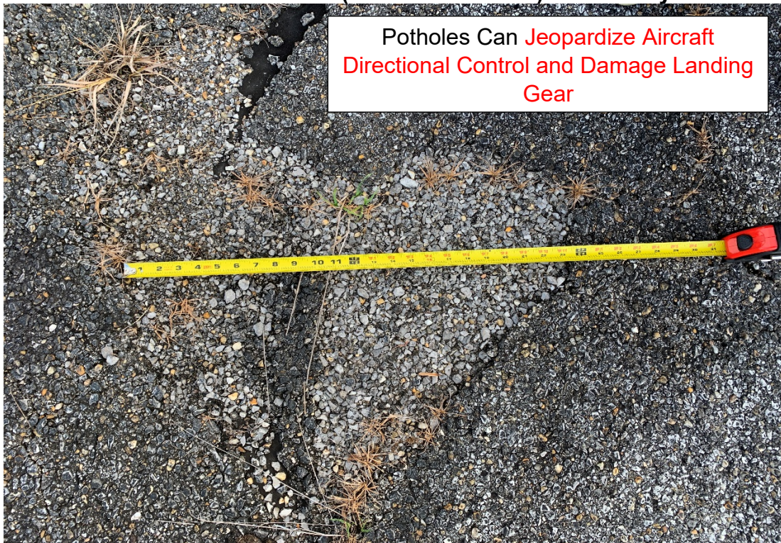
Photo #13 – Pothole (Pavement Failure) on Runway
