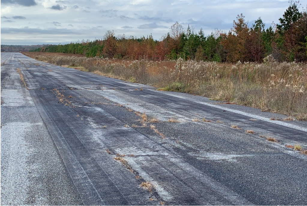
Photo #8 – Runways Light Fixtures Not Visible
