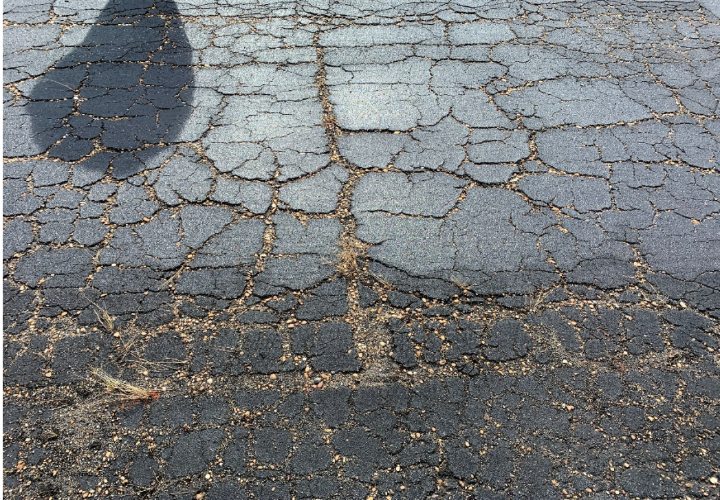
Photo #16 – Severe Alligator Cracking on Apron
