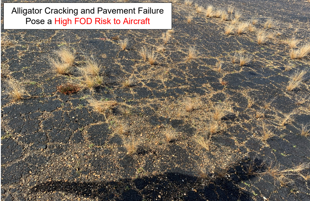
Photo #18 – Pavement Failure, Raveling, and Vegetation Growth
