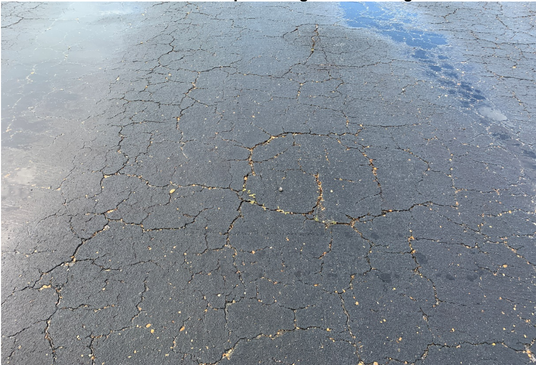
Photo #15 – Apron Alligator Cracking
