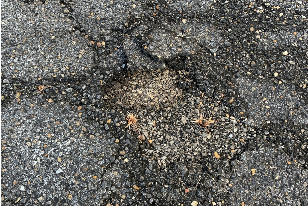
Photo #14 – Runway Pavement Failure, Exposing Underlying Layer
