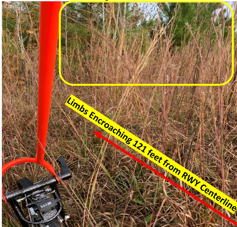
Photo #3 – Primary Surface Encroachment
