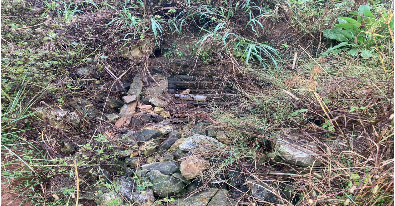
Photo #8 – Rocks and Debris on Drain Grate
