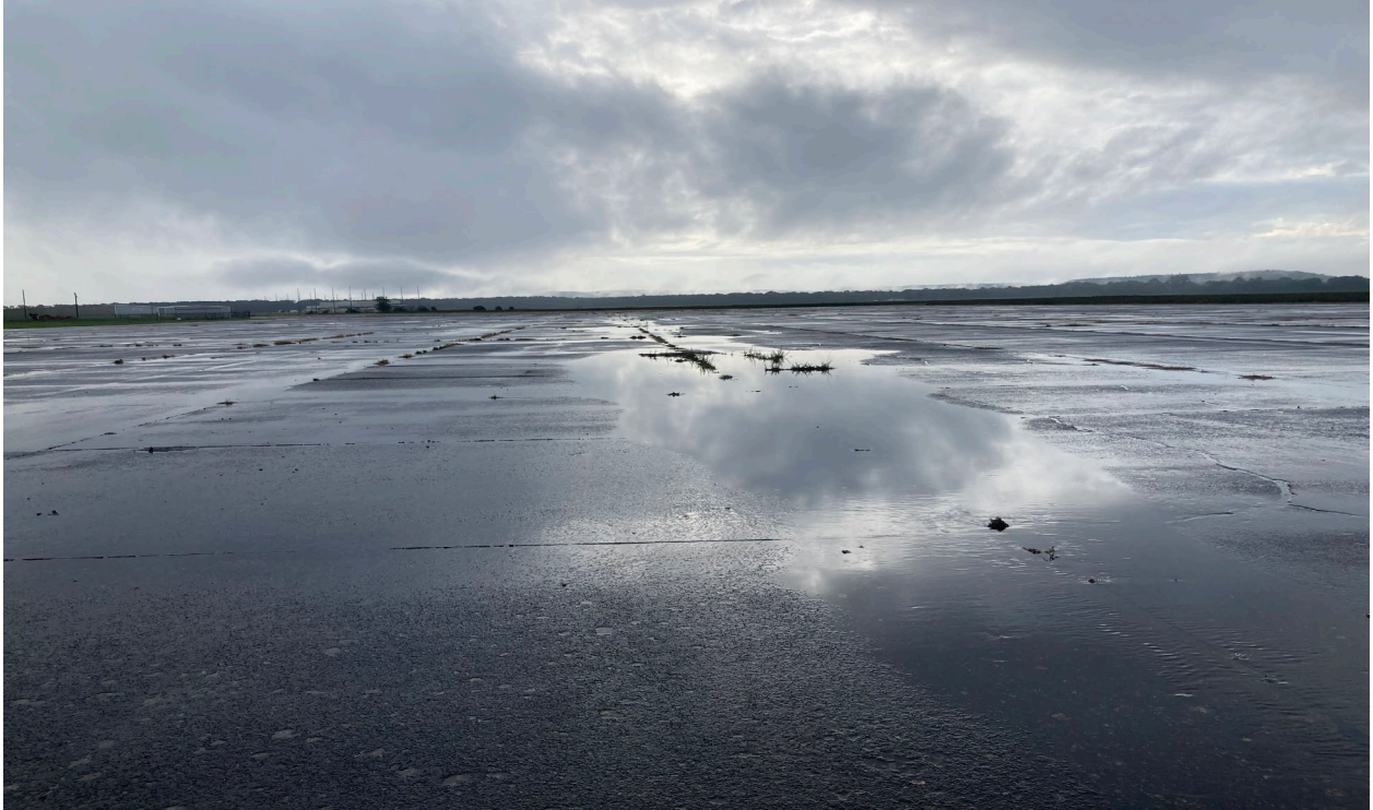
Photo #18 – Standing Water on Apron
