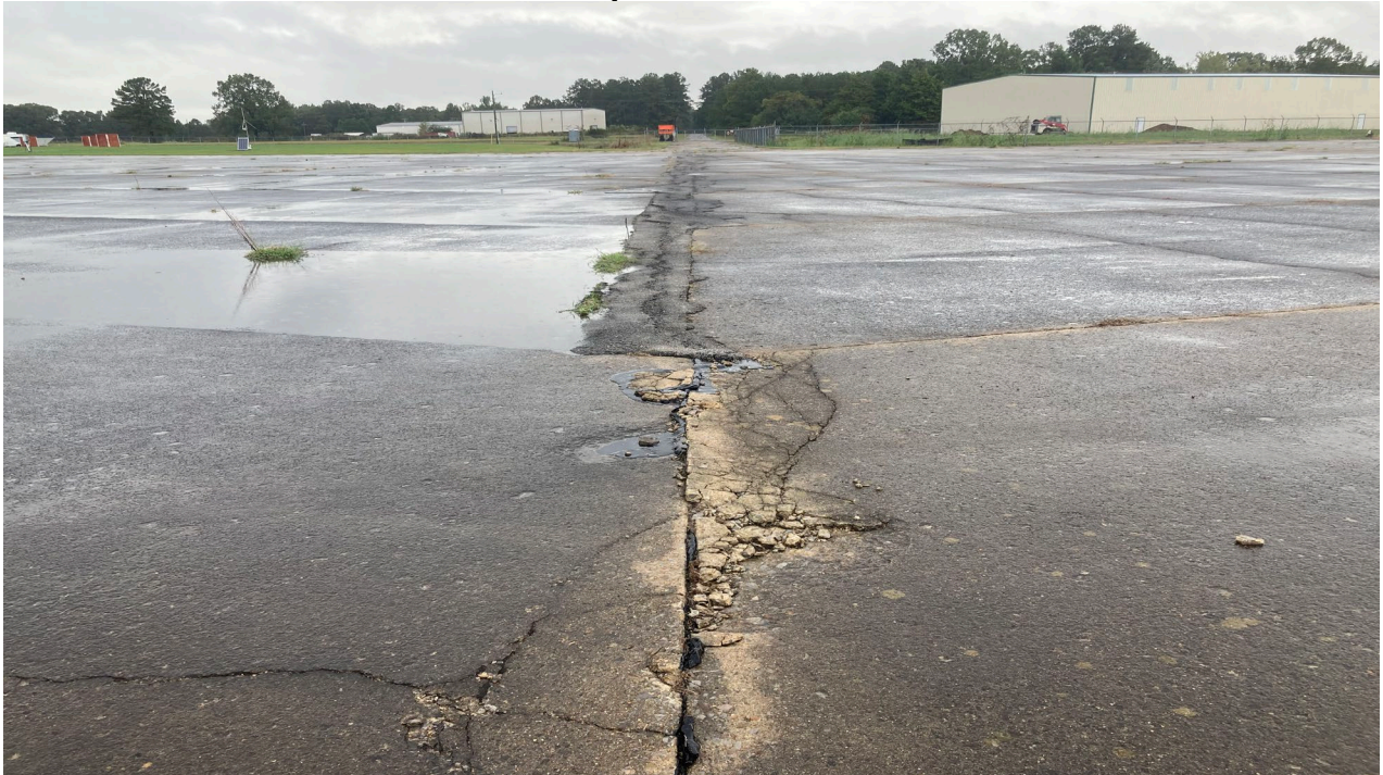
Photo #19 – Apron Pavement Failure
