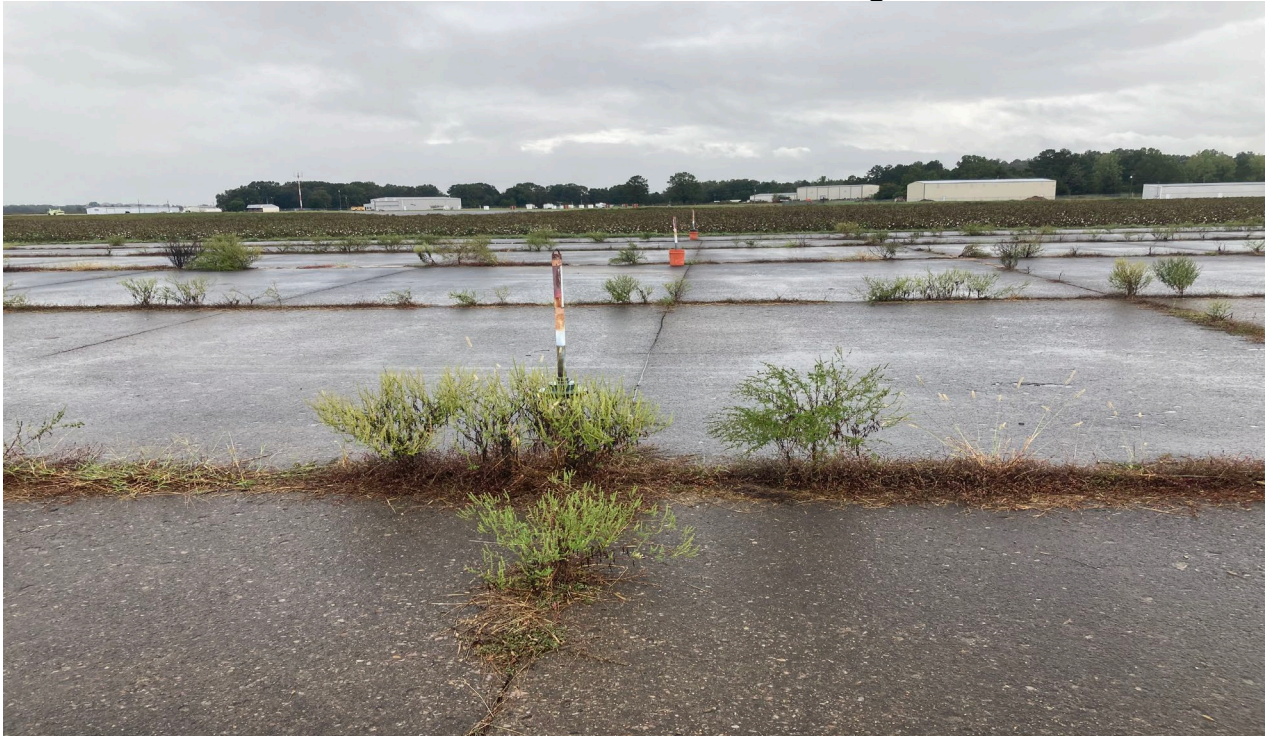
Photo #13 – Non-Standard Barricades Causing FOD Hazard
