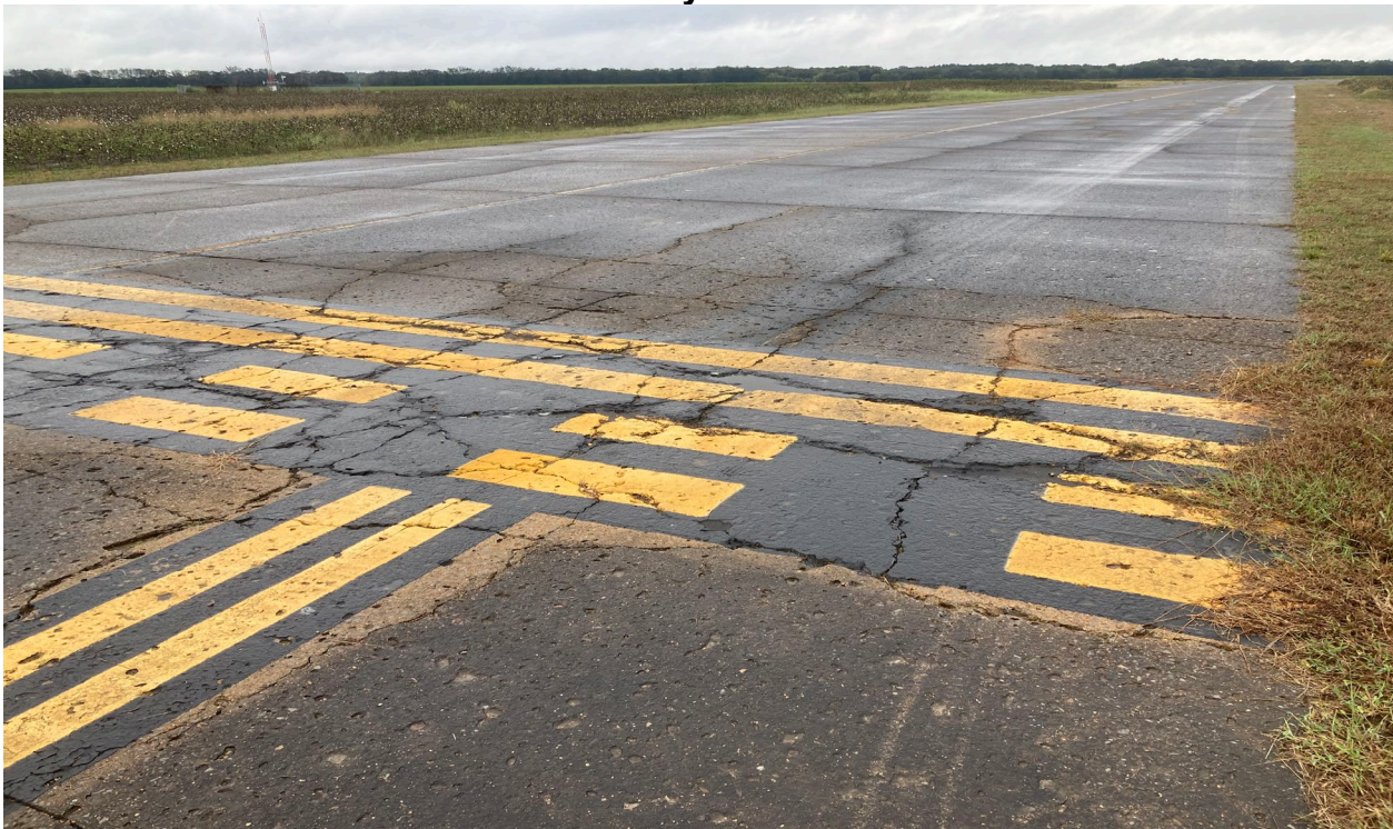
Photo #21 – Taxiway C Pavement Failure
