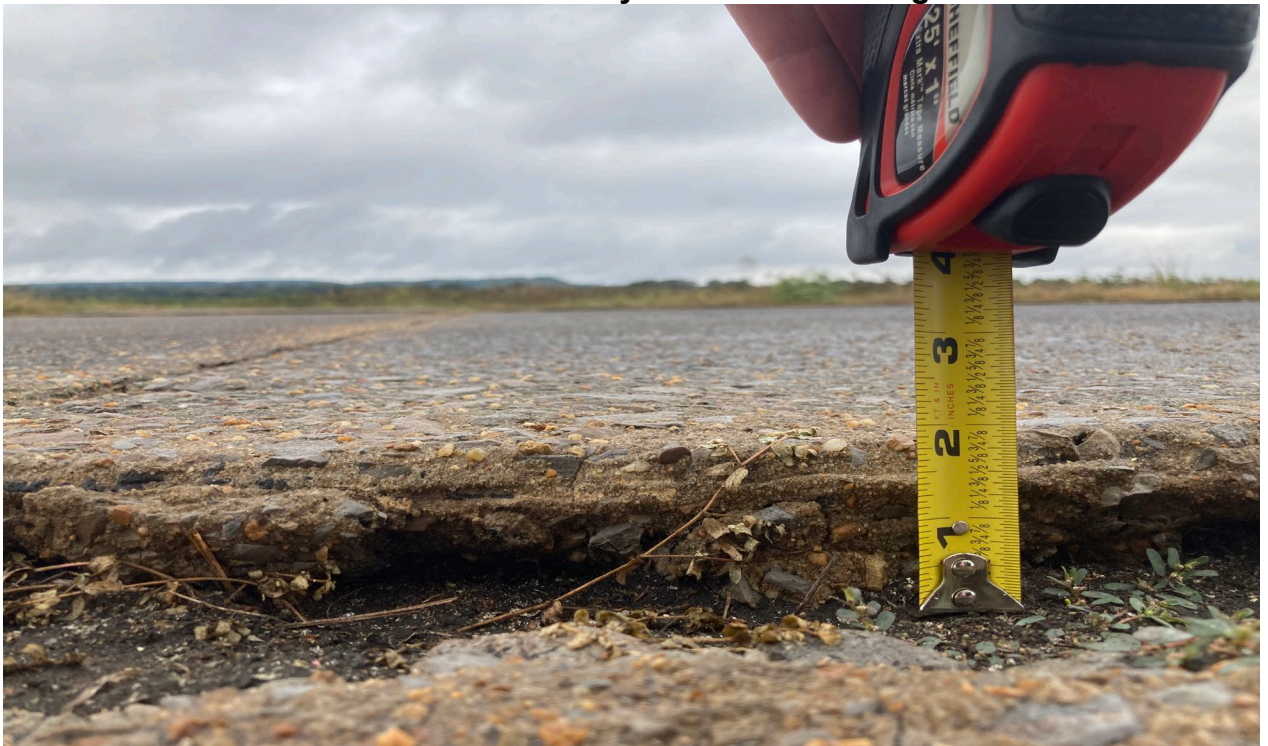
Photo #26 – Runway 18/36 Cracking
