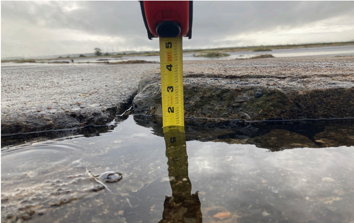
Photo #17 – Drain Slab Shift
