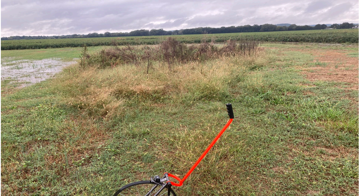
Photo #6—Hump in Runway Safety Area
