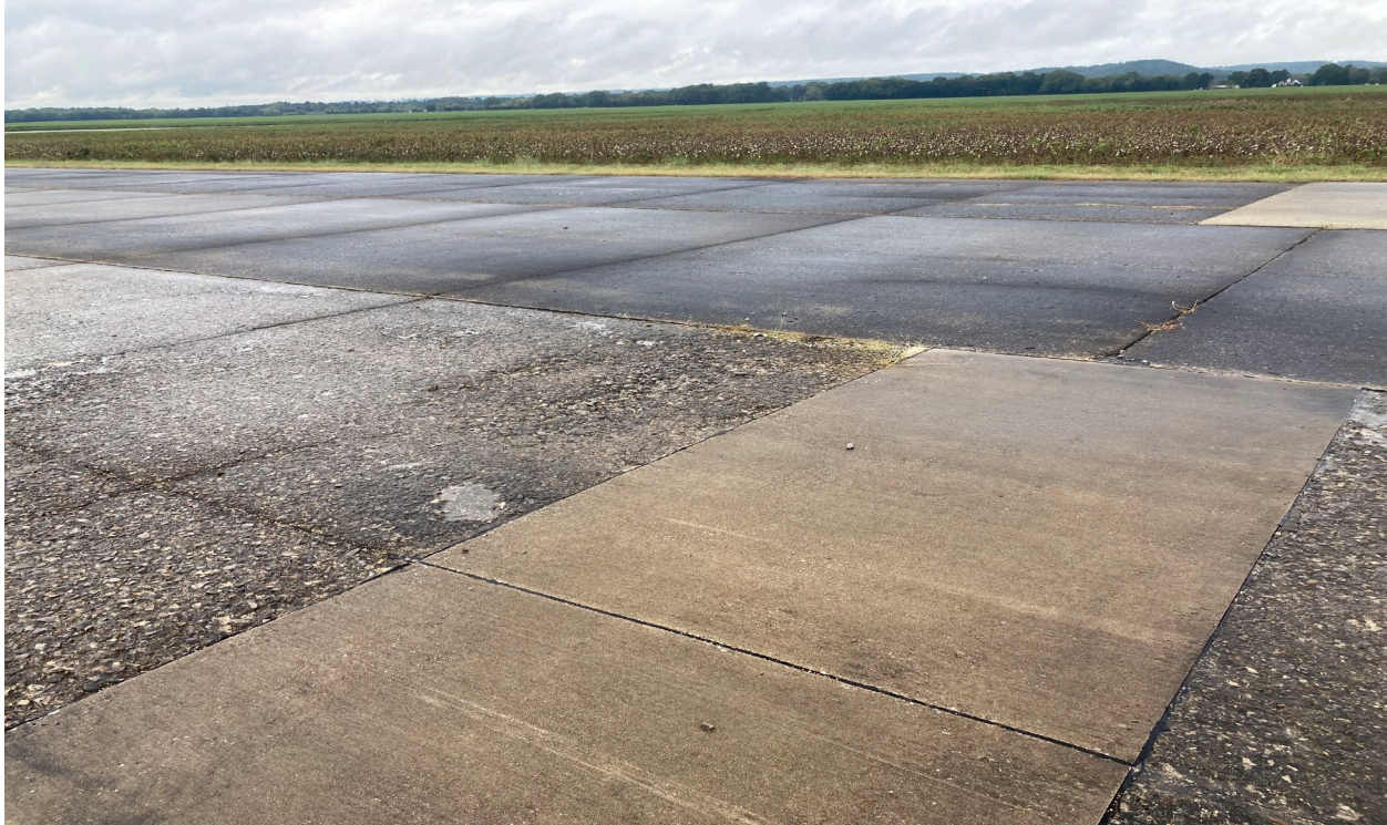
Photo #28 – Runway 18/36 Scaling and FOD
