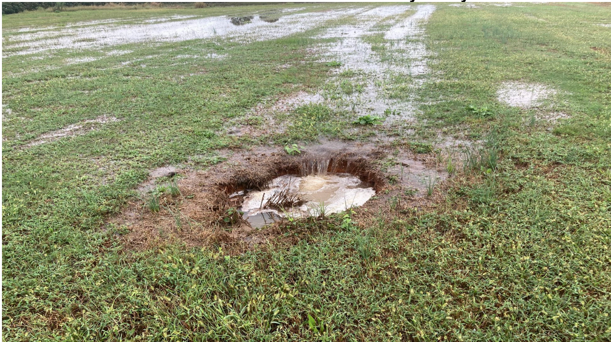
Photo #7 – Second Hole Found in Runway Safety Area
