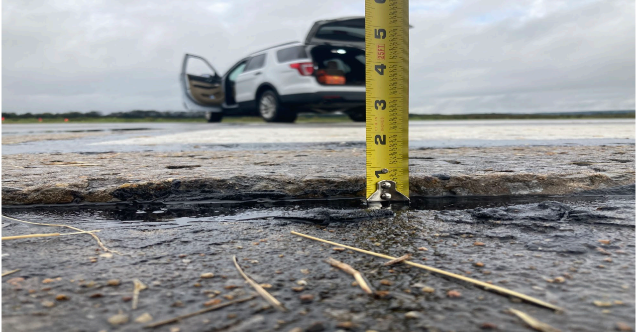
Photo #24 – Slab Shifting on Runway 13
