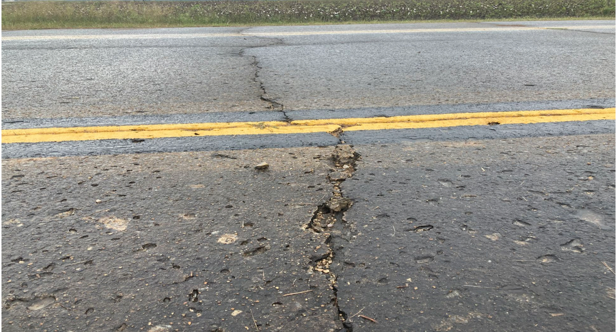
Photo #22 – Spalling on Taxiway C
