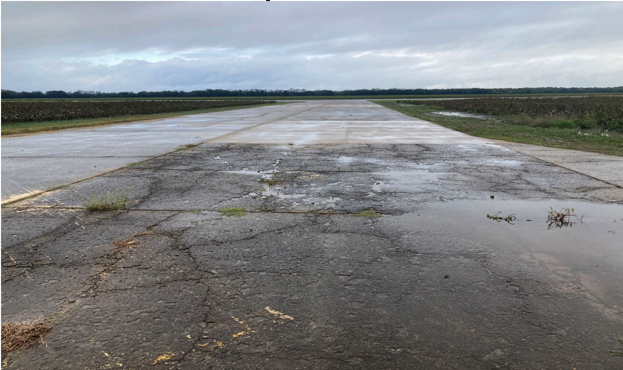
Photo # 23 – Taxiway Pavement Failure and Faded X
