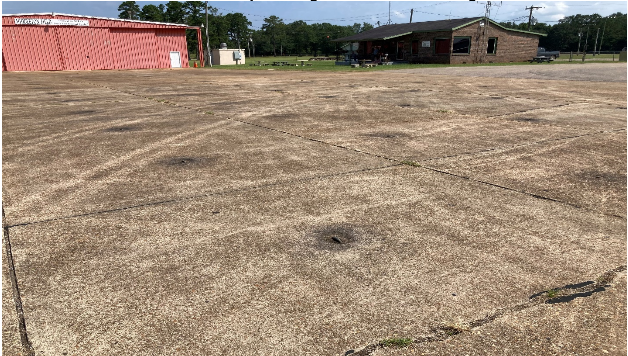
Photo #9 – Apron Vegetation and Cracking
