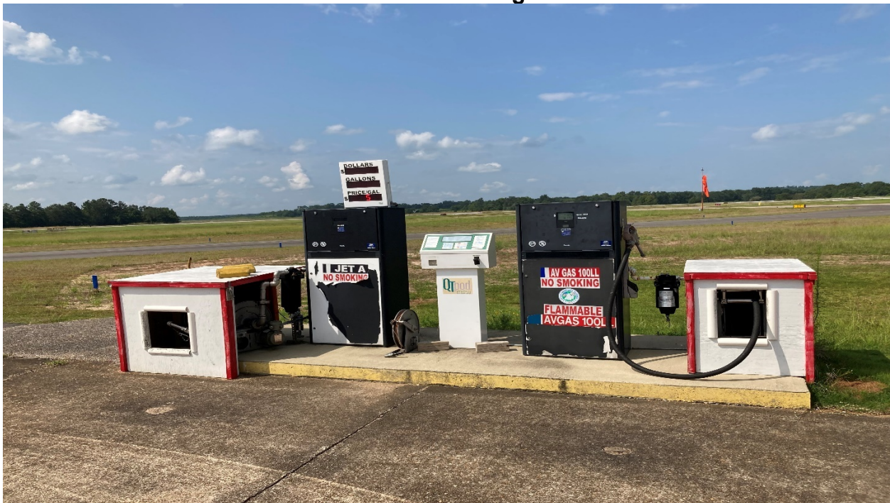
Photo #10 – Fueling Area
