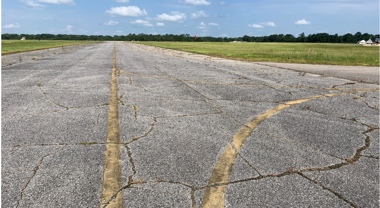
Photo #8 — RWY 10/28 Parallel Taxiway Cracking and Vegetation
