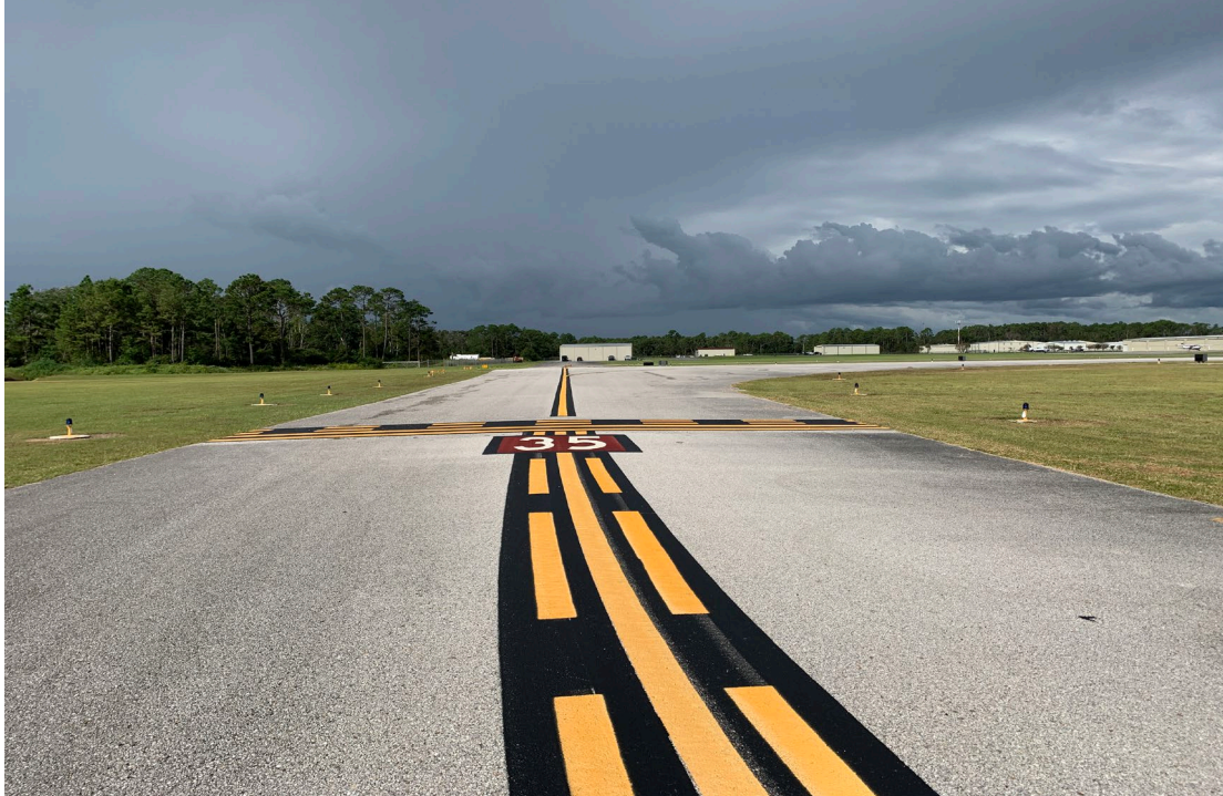
Photo #7 – Taxiway Markings
