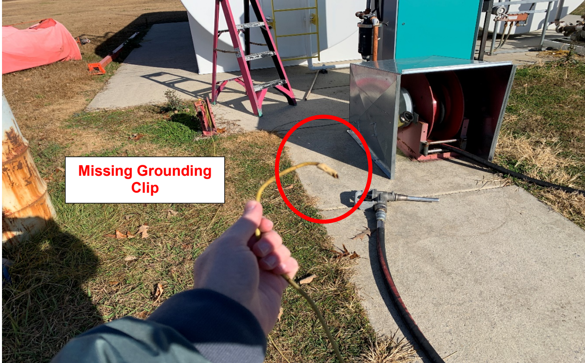
Photo #7 – Fuel Hose and Grounding Cable
