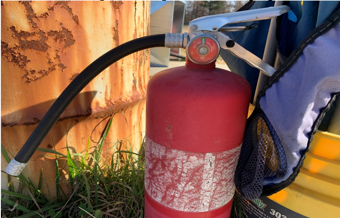
Photo #8 – Un-Charged Fire Extinguisher with Missing Tags and Labels
