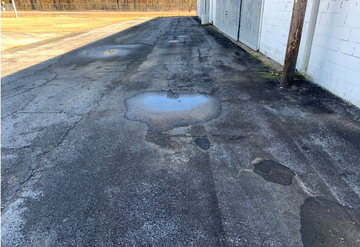
Photo #6 – Apron Cracking Near Hangars
