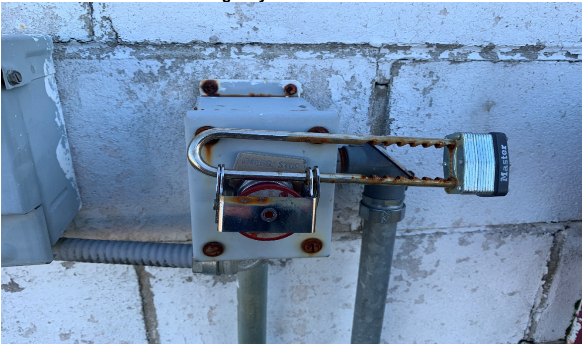
Photo #10 – Emergency Fuel Shutoff Switch with Lock
