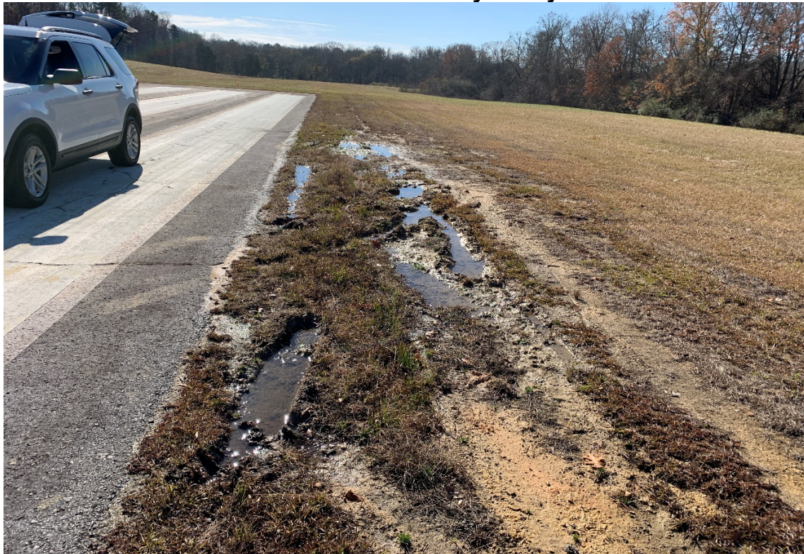
Photo #3 – Ruts in Runway Safety Area
