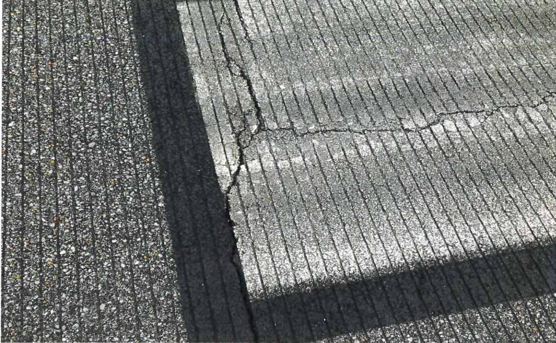
Photo # 8 – Runway Cracking
