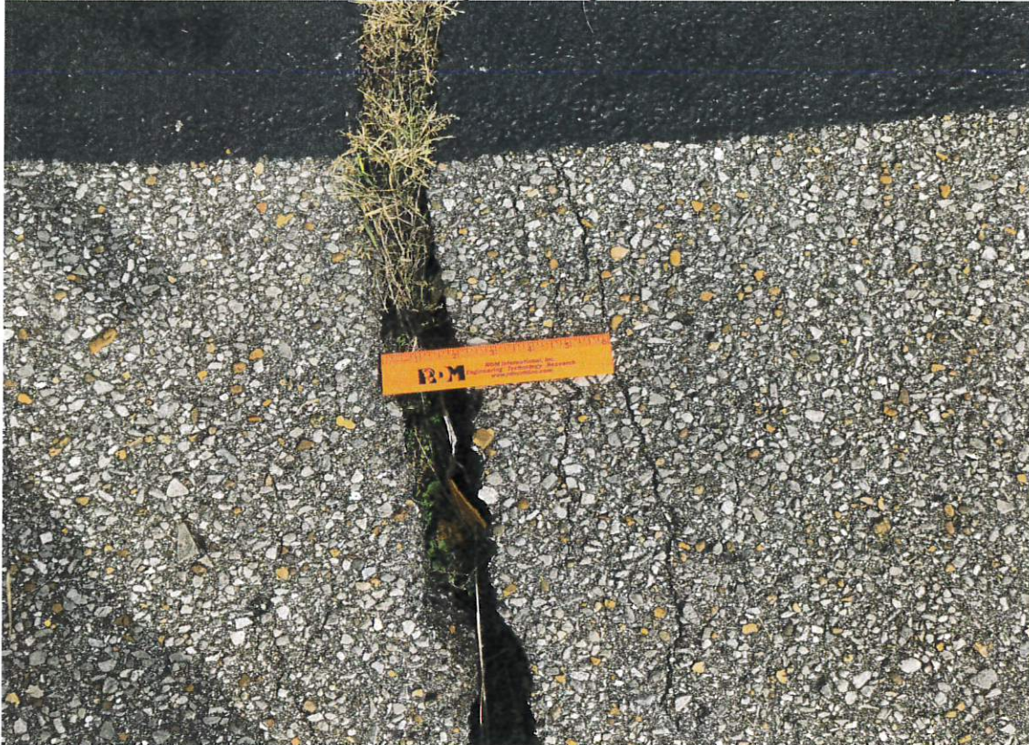
Photo # 10 – Severe Cracking with Vegetation Growth on Taxiway
