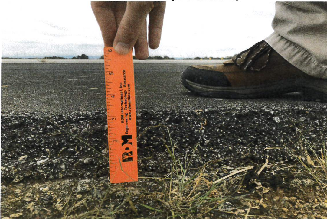
Photo #4 – Runway Pavement Lip
