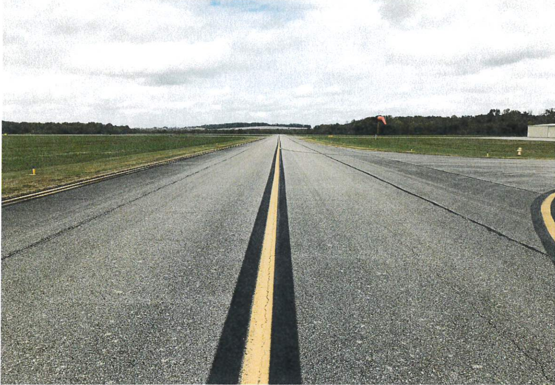
Photo #6—Taxiway Markings
