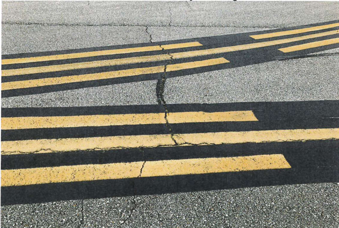
Photo # 9 – Taxiway Cracking
