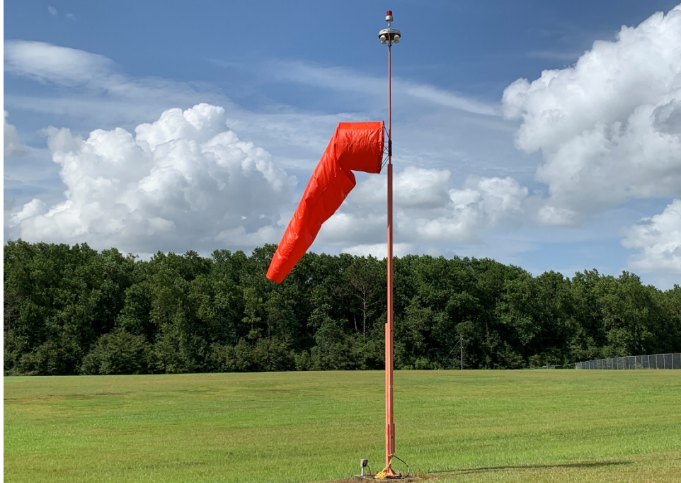
Photo # 6 – Wind Direction Indicator
