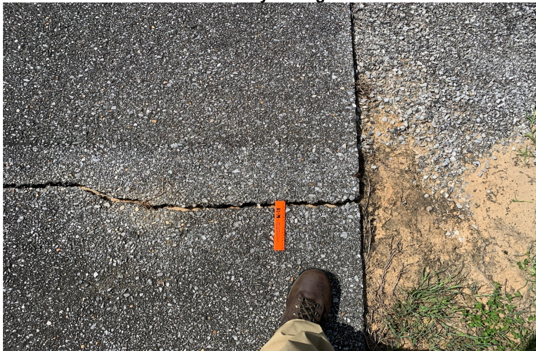
Photo #8 – Runway Paving Joint Crack
