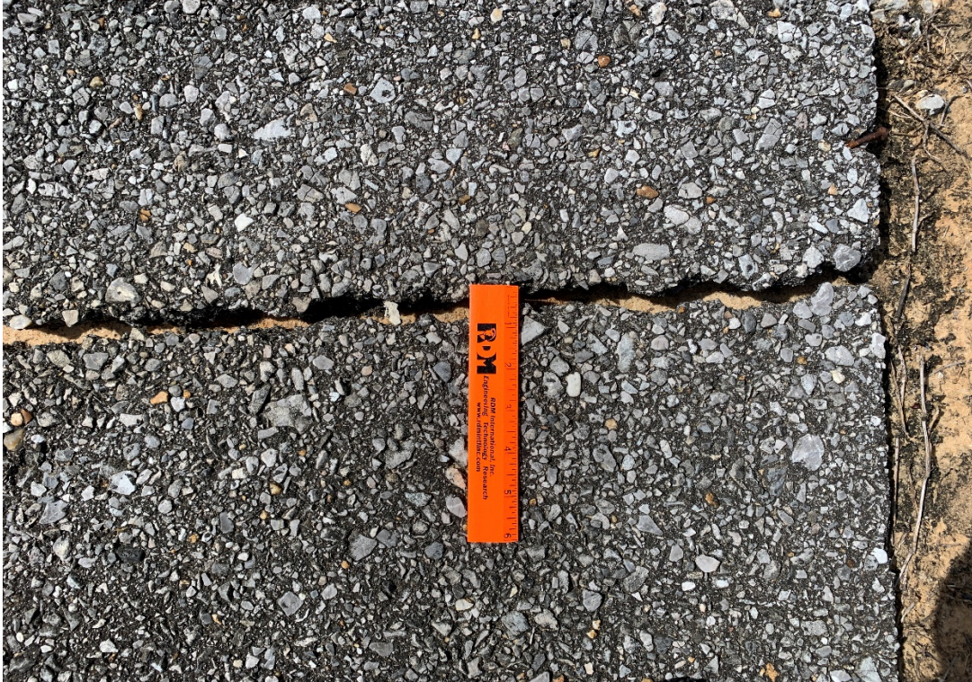
Photo #7 – Runway Paving Joint Crack
