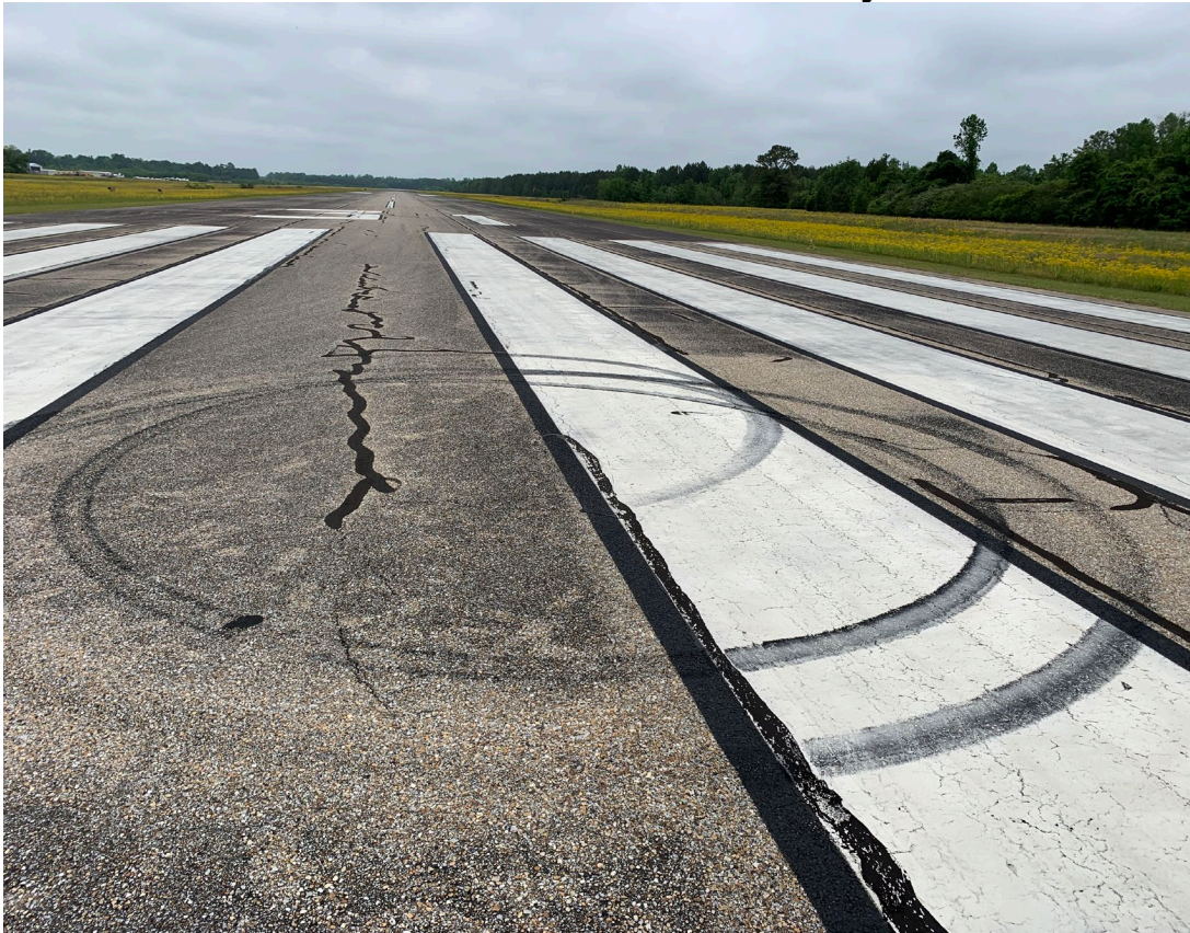
Photo #8 – Tire Marks on Runway
