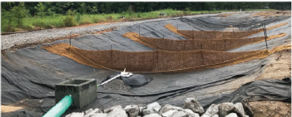
A sediment control basin which is a part of the storm water management at SR-158 extension project from Lott Road to Schillinger Road.
