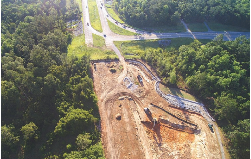
An aerial view of the SR-158 extension project from Lott Road to Schillinger Road.
