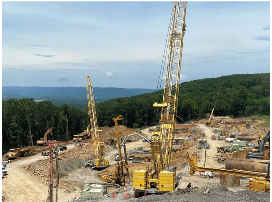
Part of the excavation and construction process to fix this portion of US-231.
