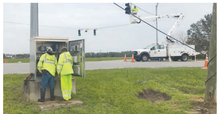
ALDOT’s Southwest Region employees closing the Bankhead Tunnel doors, removing debris and repairing traffic signals
